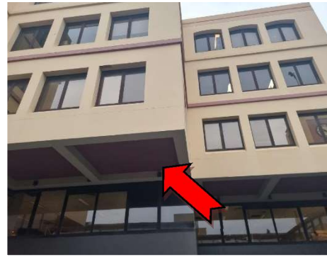
8. Exterior, level 2, courtyard soffit to level 3 offices – assumed asbestos-containing fibre cement sheeting
