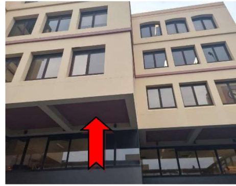
2. Exterior, level 2, courtyard soffit to level 3 offices – assumed asbestos-containing fibre cement sheeting
