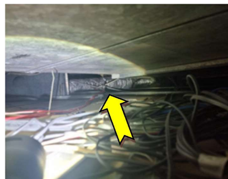
6. Interior, level 6, ceiling space, flexible ductwork – suspected SMF-containing internal insulation material
