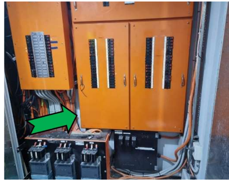
14. Interior, level 4, electrical cupboard, electrical distribution board – assumed non asbestos-containing bituminous backing board
