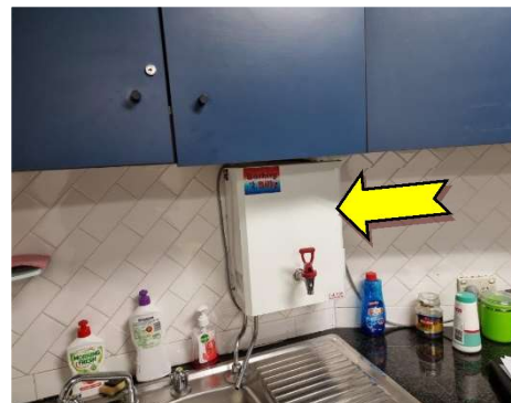
24. Interior, level 6, Harrington Lawyers tenancy, kitchen, hot water boiler – suspected SMF-containing internal insulation
