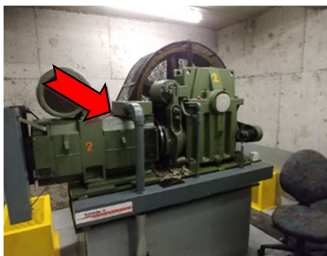
5. Interior, roof level, lift motor room, lift motor breaks – assumed asbestos-containing friction pads
