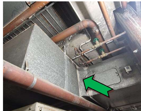
16. Interior, level 2, eastern air handling room, ductwork – assumed non asbestos-containing mastic sealant
