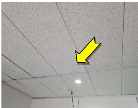
25. Interior, level 5, eastern elevation, throughout Invast Global tenancy, ceiling – suspected SMF-containing compressed ceiling tiles
