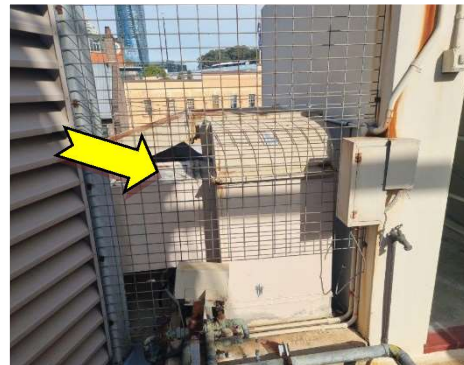
22. Exterior, roof level, throughout, rigid ductwork – suspected SMF-containing internal insulation material
