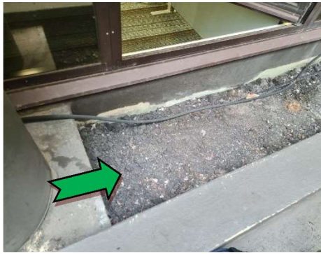
7. Exterior, level 2, courtyard, within garden beds – non asbestos-containing fibre cement debris
