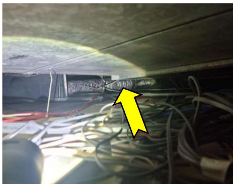
23. Interior, level 6, ceiling space, flexible ductwork – suspected SMF-containing internal insulation material
