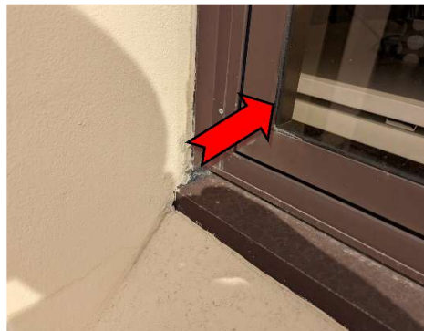
6. Exterior, level 2, eastern elevation, windows– asbestos-containing mastic material
