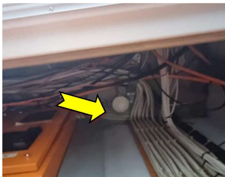
27. Interior, level 4, electrical cupboard, ceiling and floor penetrations, pillow insulation – suspected SMF-containing insulation material
