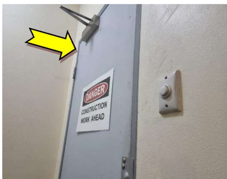
29. Interior, level 2, throughout, fire doors, door frames – lead-containing blue (light) upper paint system
