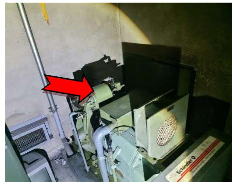
4. Interior, lower B2 level, lift motor room 3, lift motor breaks – assumed asbestos-containing friction pads
