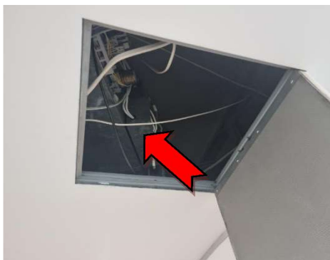
11. Interior, level 6, within ceiling space, air handling unit, heaterbank – assumed asbestos-containing millboard insulation
