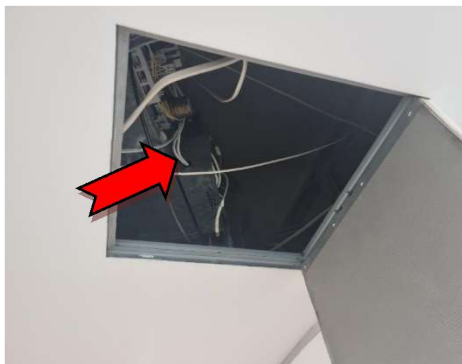
3. Interior, level 6, within ceiling space, air handling unit, heaterbank – assumed asbestos-containing millboard insulation
