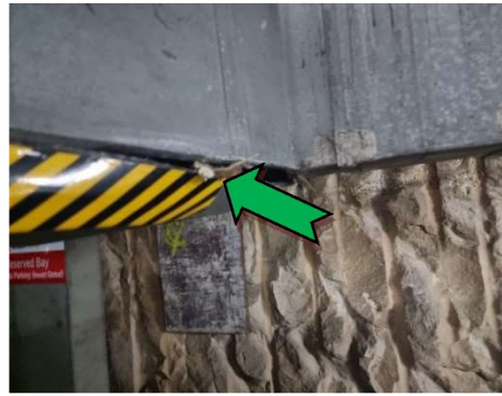
20. Interior, upper B1 level, adjacent carpark entrance, rigid ductwork – non asbestos-containing internal insulation
