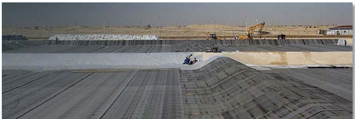
Figure 3-2: An example of a bituminous geomembrane lining system being applied to a reservoir. Source: Coletanche.
