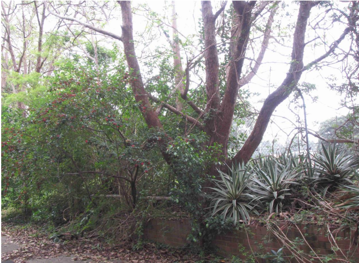
Figure 30 Shows the existing brick retaining wall that ensure no structural or woody roots will be impacted/cut as part of these works as per Section 10.2.1 Typical diagram of adjoining tree and retaining wall.
