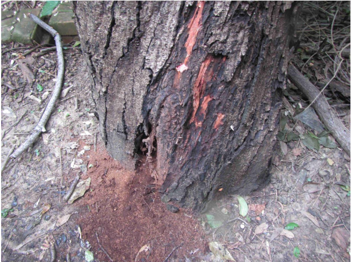
Figure 36 Shows Tree 206 lower base with extensive borer damage on a lean.
