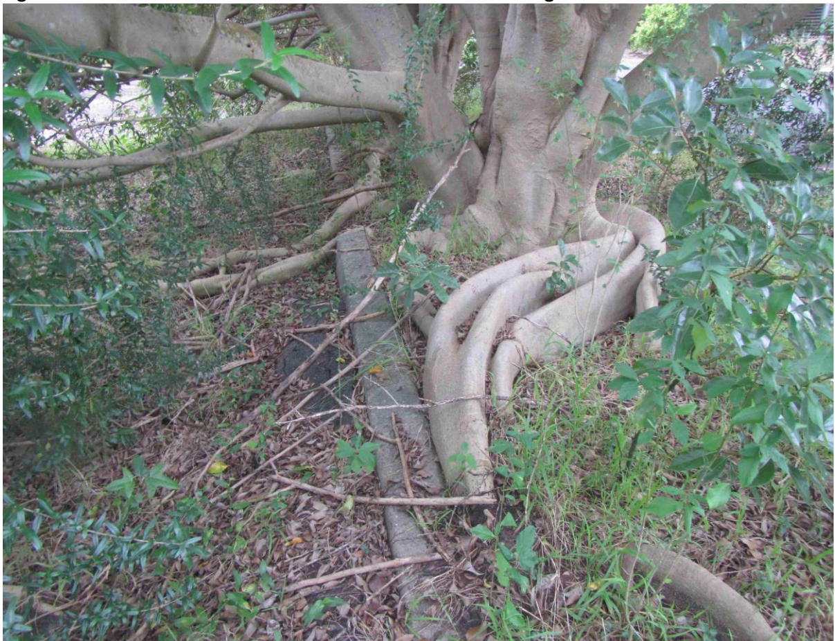
Figure 37 Shows the fig trees that have overgrown the carpark planter box.
