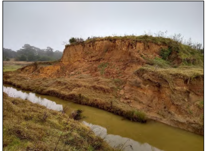
Plate 4 – View south west of breached dam wall.
