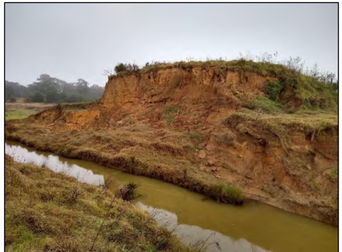
Plate 4 – View south west of breached dam wall.
