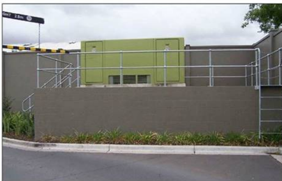
Figure 51 - Example substation raised above 1:100 flood level
