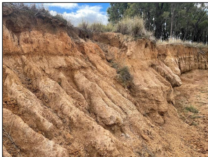
Plate 4: Severe gully erosion associated with White Creek.
