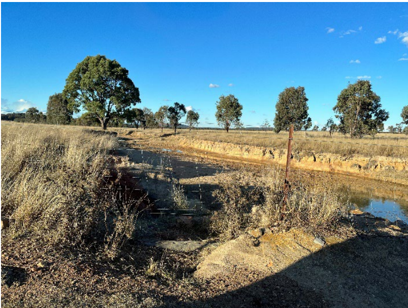
Photograph 6.4 Localised gully erosion contributing to bank instability
