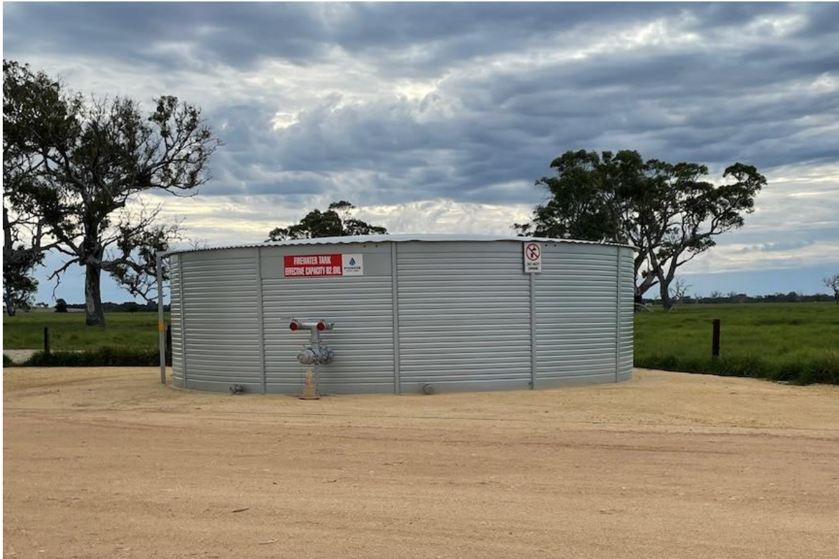
Plate 2: Example of community water storage for bushfire protection
