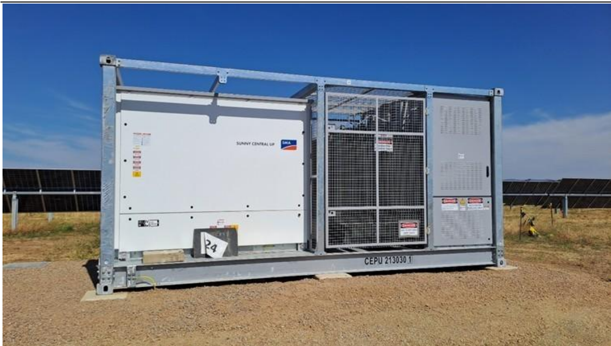
Plate 2: PCU at Glenrowan Solar Farm (source: Pacific Partnerships, 2025)
