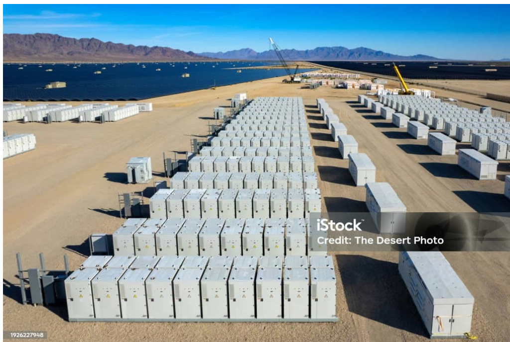
Figure 3-3 Electrical storage array at solar power plant stock photo (iStockphoto, 2025)
