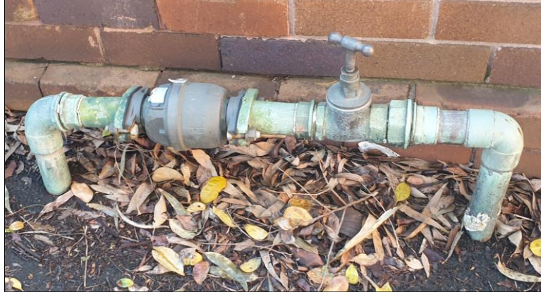
Fig 3.2 – Main Water Meter
