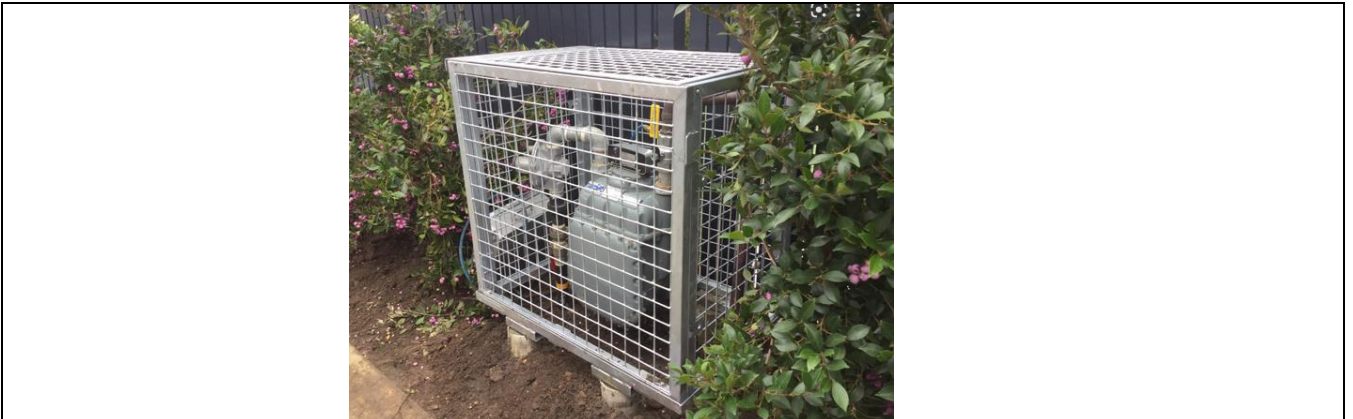
Image 7, Natural Gas boundary meter, regulator & enclosure
