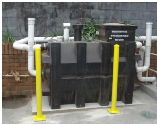
Image 10, Example of an Above ground Grease Arrestor displayed for fitting example. Below ground grease arrestors are preferred.
