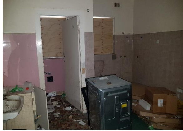
Figure 4.12 Bathroom on the ground floor with heavy debris and boarded windows.
