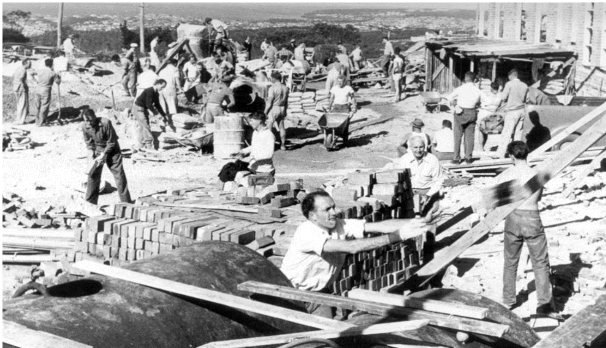
Figure 3.6 Volunteer workers helping with the construction of McLeod House, c1957. (Source: ‘Nothing is Impossible: Adventures in cerebral palsy’ by Neil McLeod, 1986)
