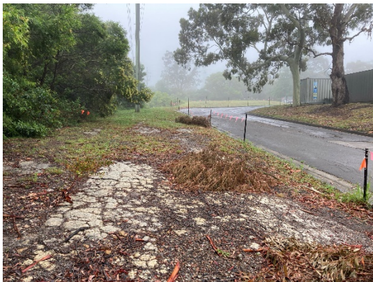
Figure 4.3 Degrading bedrock, facing north. (Source: GML, 2020)
