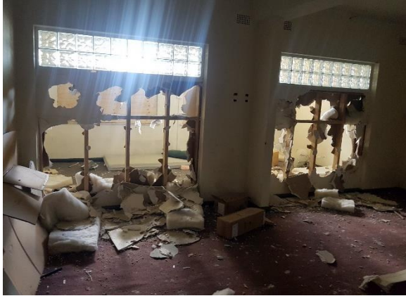
Figure 4.11 Partially demolished walls and debris caused by vandalism.
