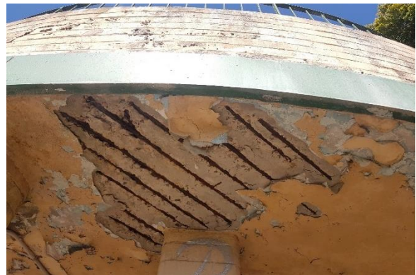
Figure 4.4 Concrete cancer to the underside of the first-floor verandah.
