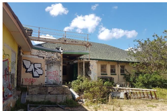
Figure 4.6 Partially demolished walls and broken roof tiles to one of the wings.
