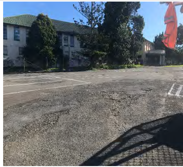
Photograph 1: View of the eastern carpark, cracks and holes observed on bitumen pavement.
