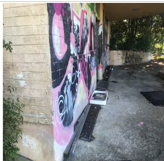
Photograph 14: Drain adjacent to the western workshop entry.
