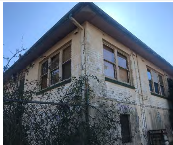
Photograph 3: Asbestos eaves observed on building structures.
