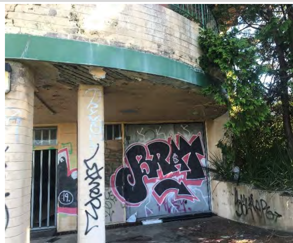
Photograph 11: Flaking paint observed in poor condition on the eastern building.
