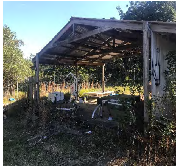
Photograph 5: Shed on the north western side of the site, scrap materials and redundant fridge noted.
