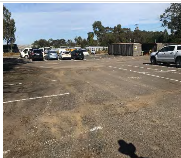
Photograph 15: View of central car park to the west. Bitumen pavement observed in poor condition with cracking, holes and oil staining.
