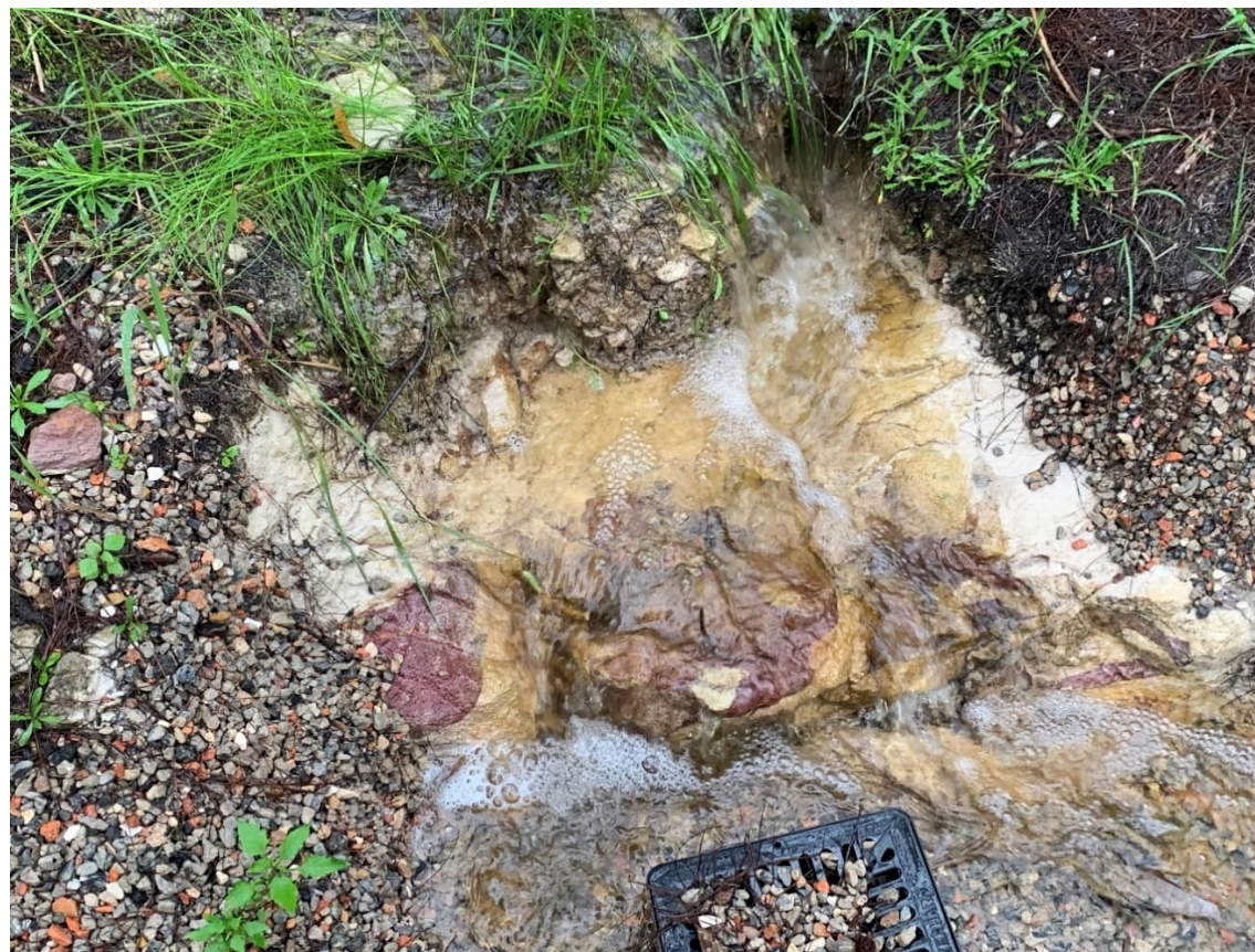
Figure 6: Overland flow from lower embankment into 150mm diameter pit discharging into Arranounbai School driveway
