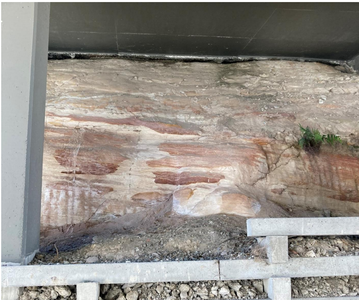
Figure 3: Exposed rock cutting below walkway
