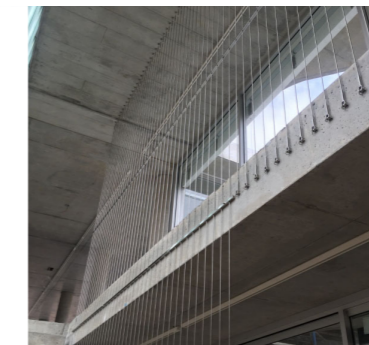
SCR 01 - FALL PREVENTION BARRIER TENSILE VERTICAL CABLE SYSTEM ALONG CORRIDOR AND RAMPS
