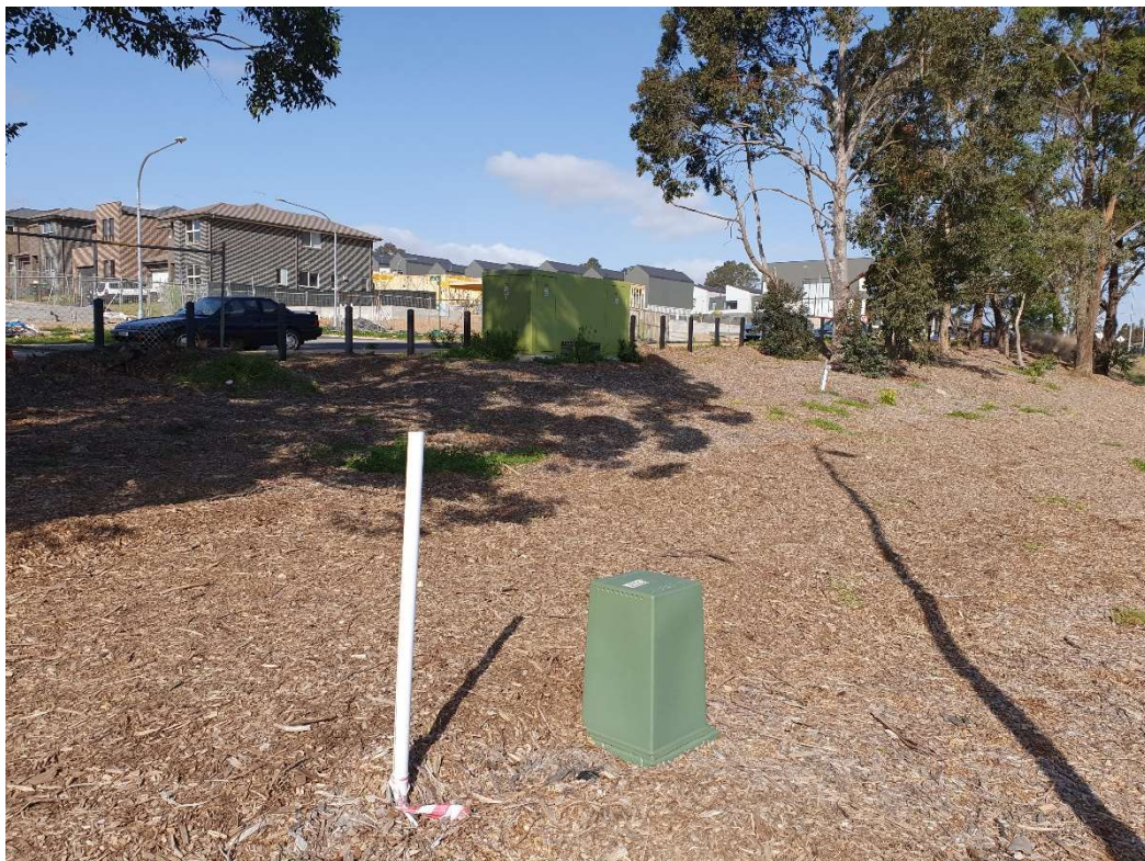
Figure 3.2: Existing electrical pillar along Stone Mason Drive(between the kiosk and Telstra Tower)
