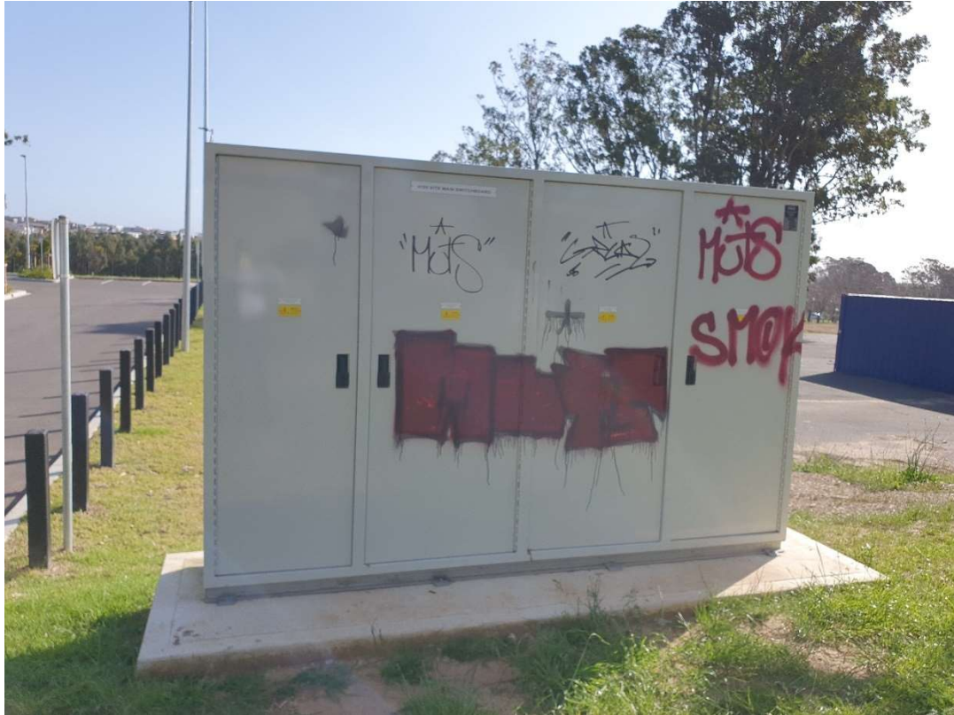
Figure 3.3: Existing main switch board
