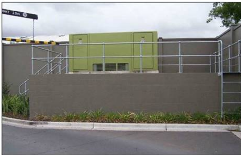
Figure 51 - Example substation raised above 1:100 flood level
