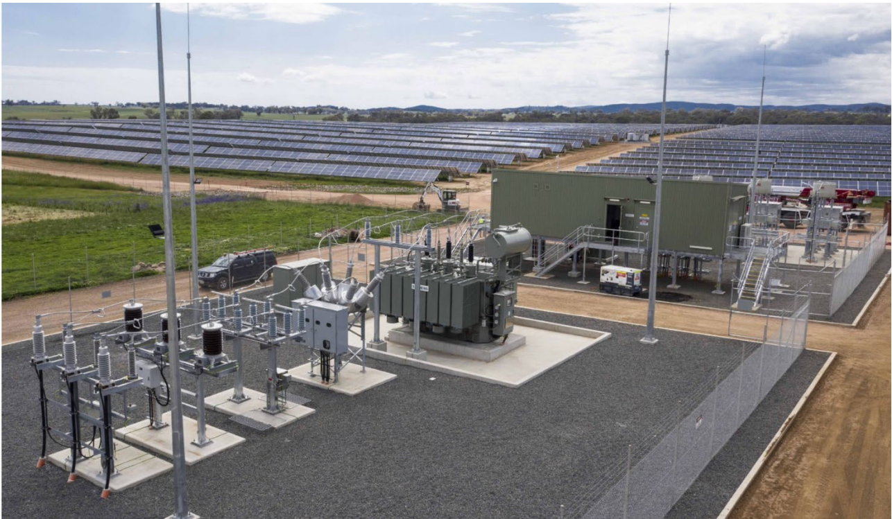
Figure 3-5 Typical substation; Molong Solar Farm (33/66kv connection).
