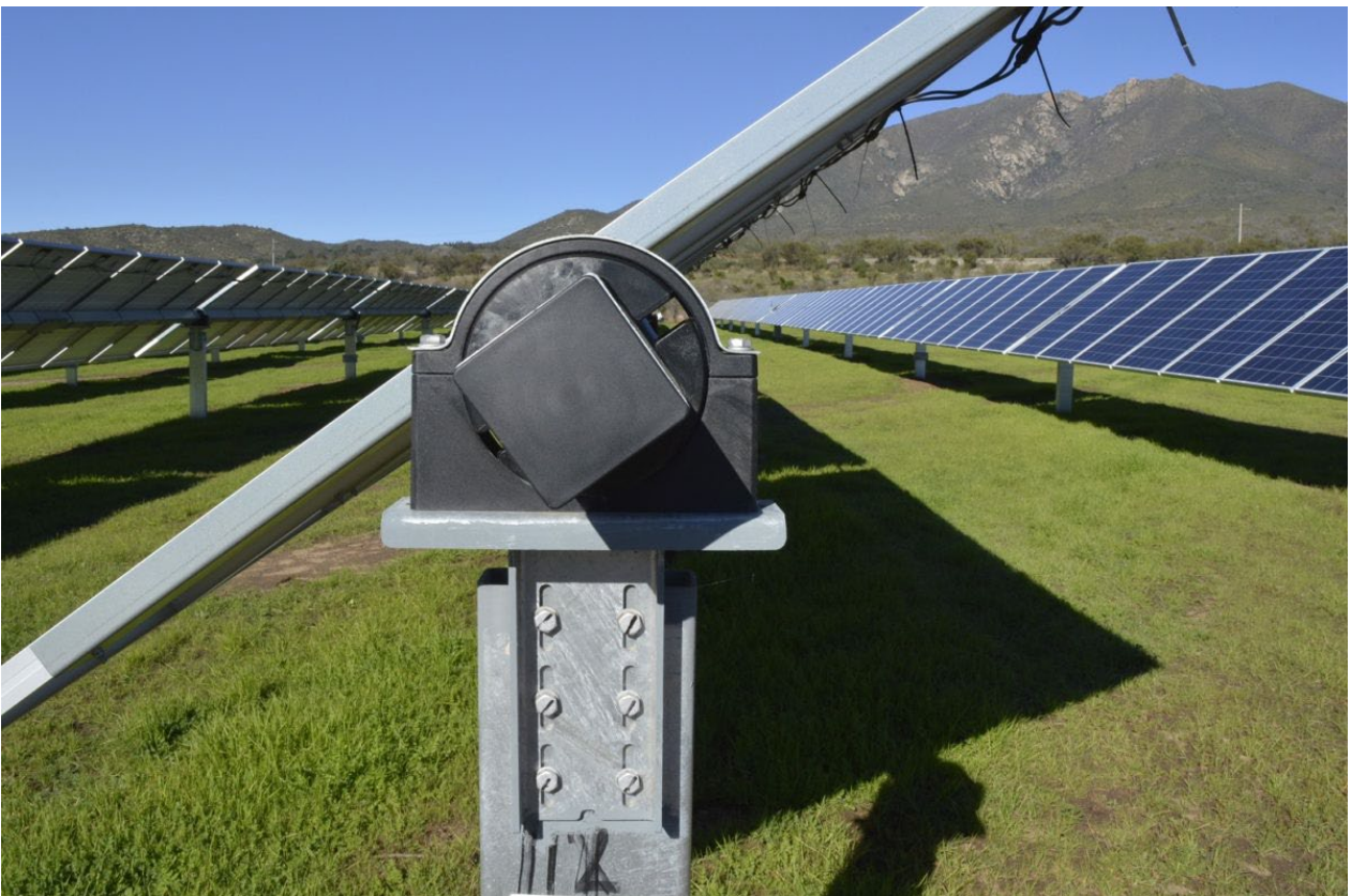
Figure 3-2 Typical solar array and mounts in operation Close up on tracker systems with solar modules mounted (Source: Shutterstock image)
