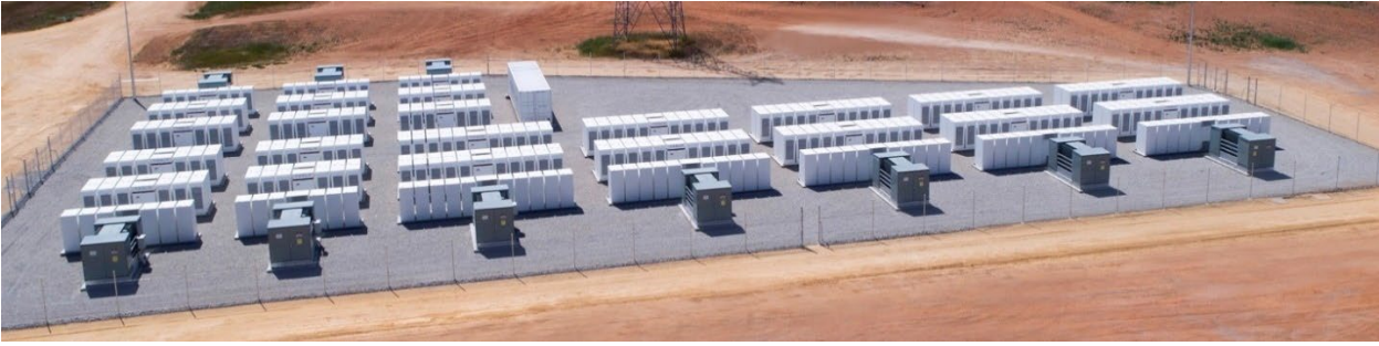
Figure 3-3 Illustrative example of BESS (Gannwarra BESS 50MWh using Tesla Megapack Technology; source: https://www.energyaustralia.com.au/about-us/energy-generation/gannawarra-battery-storage )
