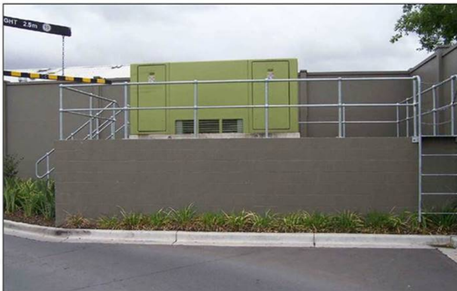
Figure 51 - Example substation raised above 1:100 flood level
