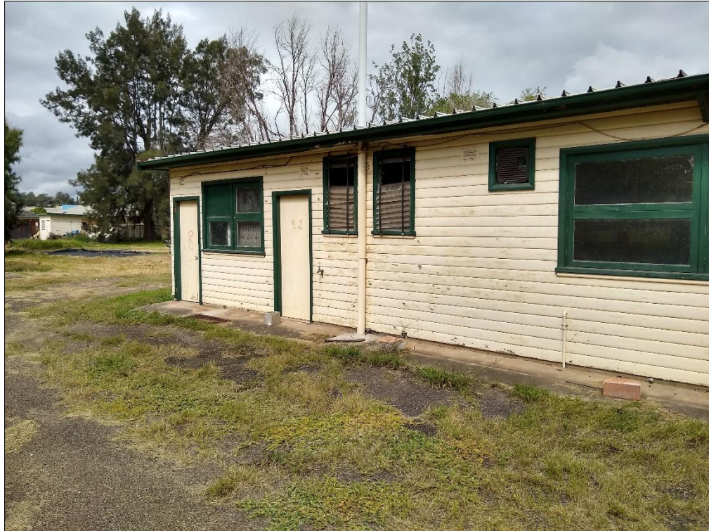
Figure 21: Surface area found along the north eastern face of Building 8.
