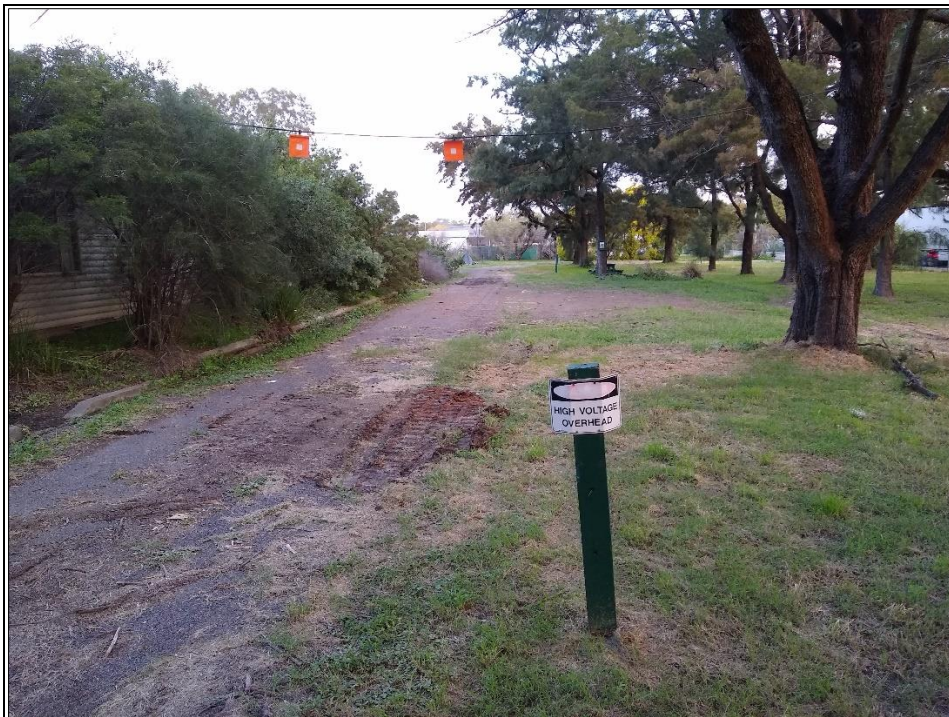
Figure 4: General condition of asphalt access track, south of the buildings, looking east.
