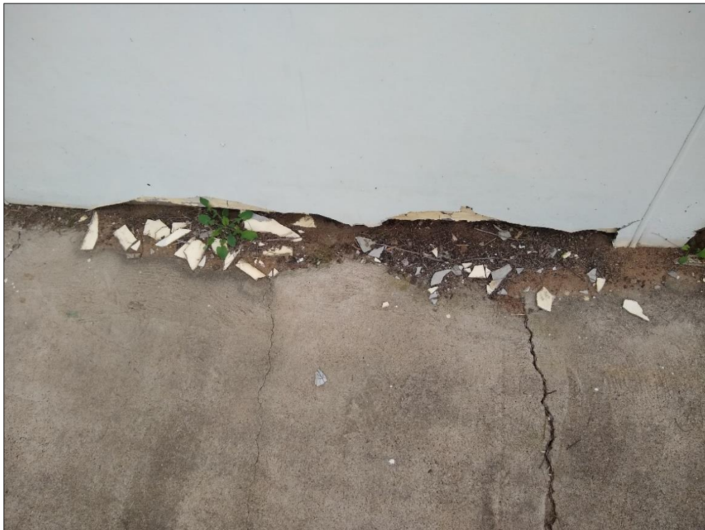
Figure 32: Damaged external wall located along the southern face of Building 6. Sampling location for fibro sample F5/JRK.
