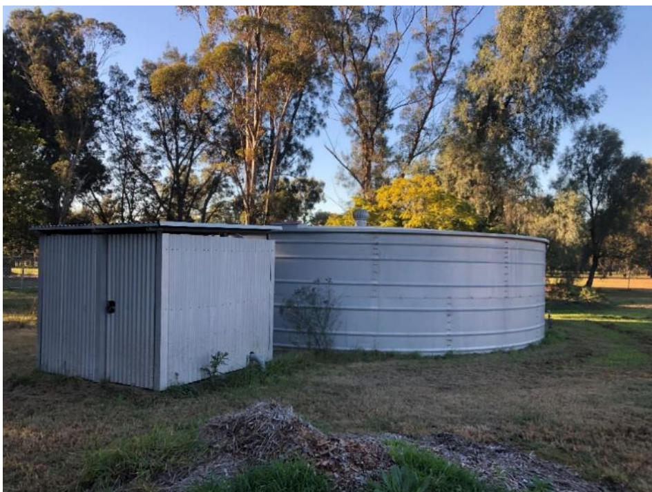
Photograph 19: Galvanised water tank.
