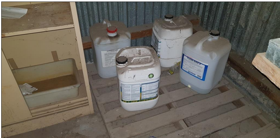
Figure 7: Stored chemical containers within the Hazchem building.
