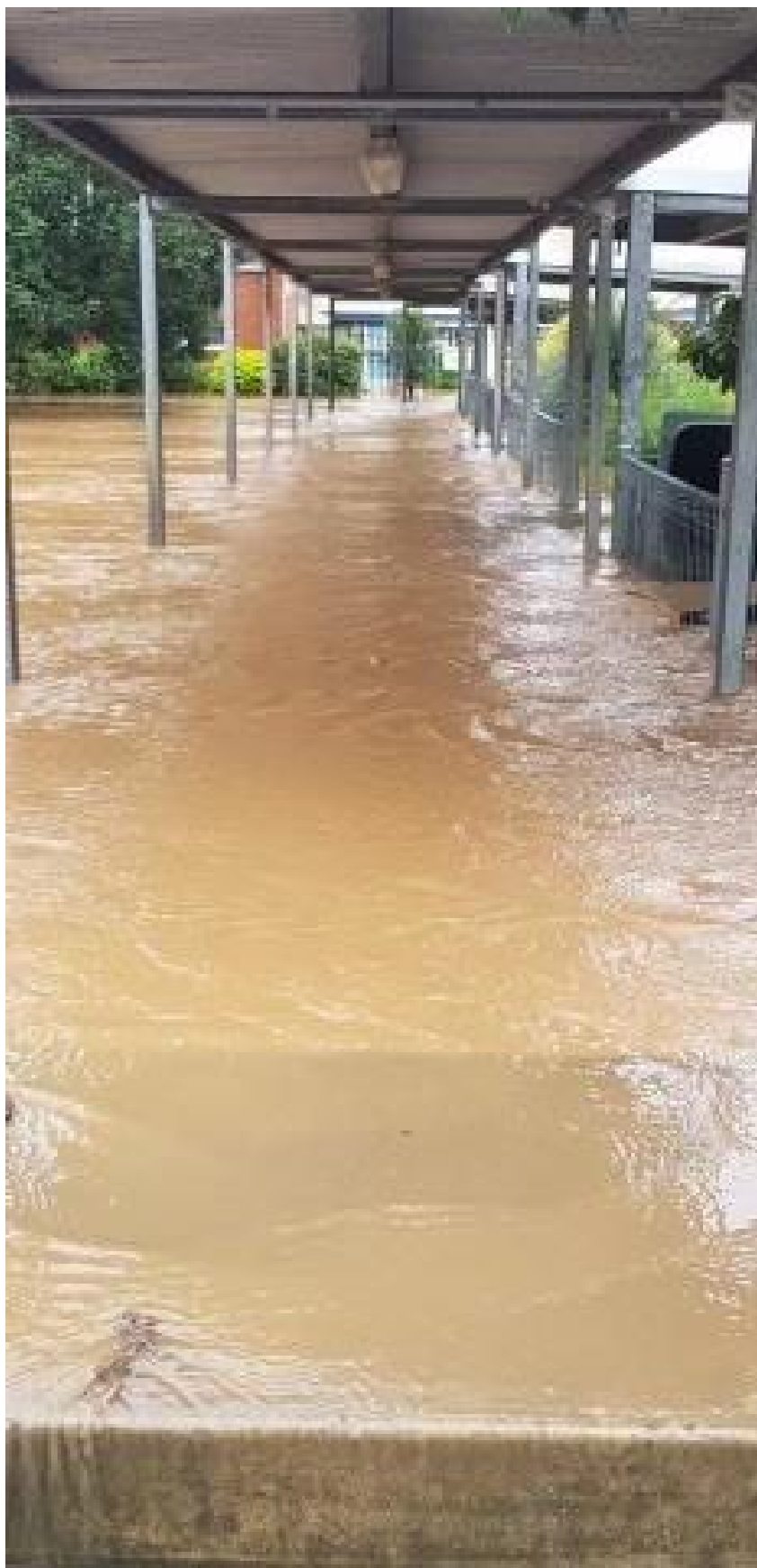
MEPS access flood impacted
