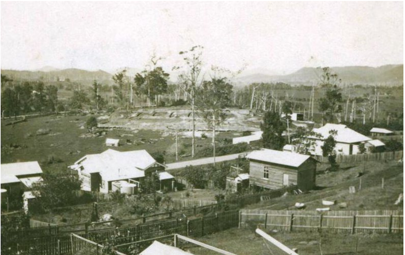
Plate 3.2 From Hartigan's Hill looking across to Riverview Street showing commencement of construction initial earthworks works on Hartigan's Estate for the future Murwillumbah High School. c. 1928. Source: M19-34, Tweed Regional Museum archives. Photographer Unknown.
