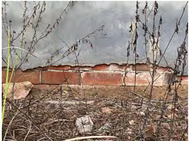
Plate 7.8 Mid-twentieth century extension at point of intersection with original structure. Source: EMM 2021.
