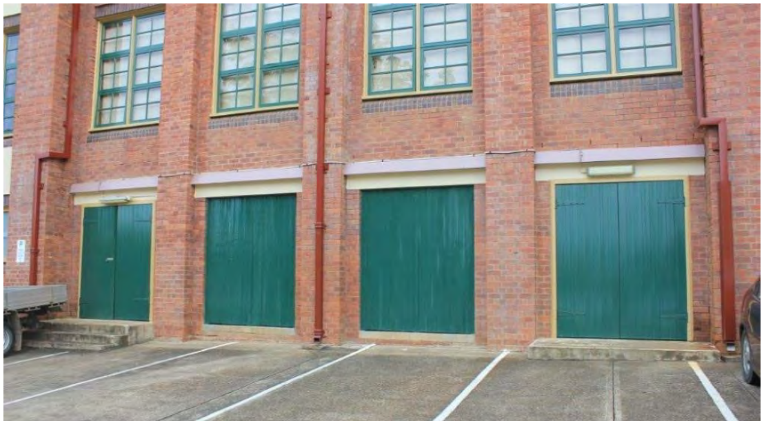
Plate 5.6 View of the lower portion of Block A with entry ways to basement level. Source: EMM 2021.
