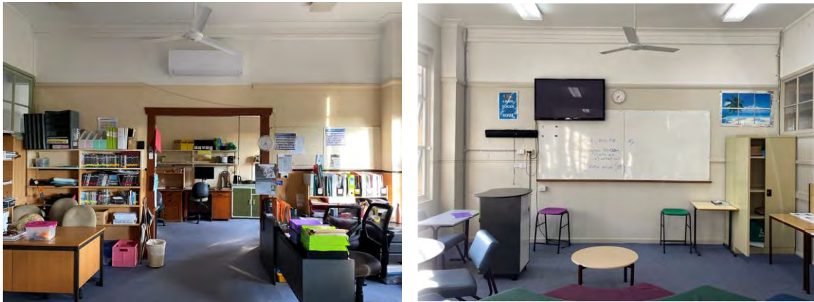
Plate 9.5 Original wall fabric to staff room A21 (left) and classroom A19 proposed for demolition. Source: EMM 2021.
