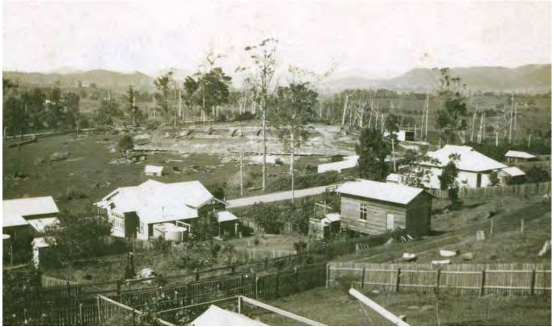
Plate 4.5 From Hartigan's Hill looking across to Riverview Street showing commencement of construction initial earthworks works on Hartigan's Estate for the future Murwillumbah High School. c. 1928. Source: M19-34, Tweed Regional Museum archives. Photographer Unknown.
