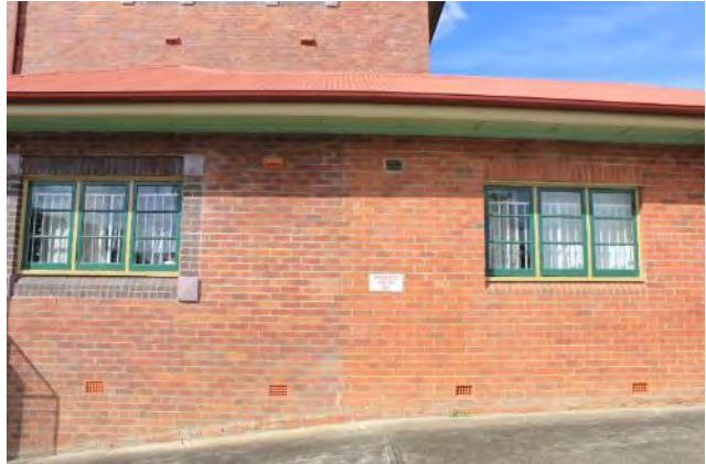
Plate 7.2 Mid-twentieth century extension at point of intersection with original structure. Source: EMM 2021.
