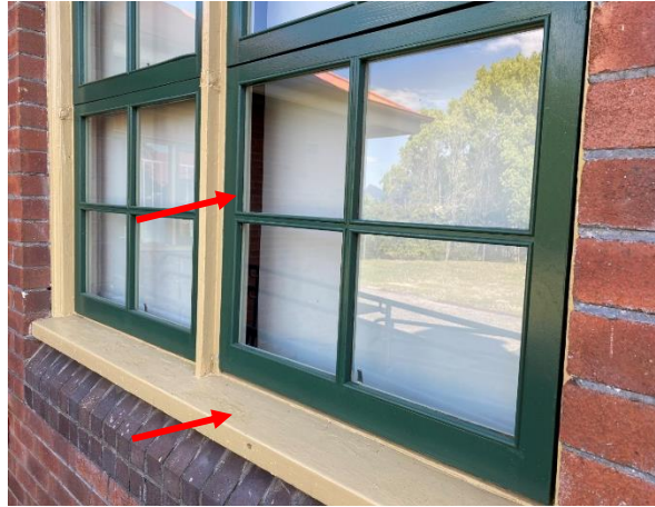
Photo 2: Building A - Lead based green and yellow timber window frames
