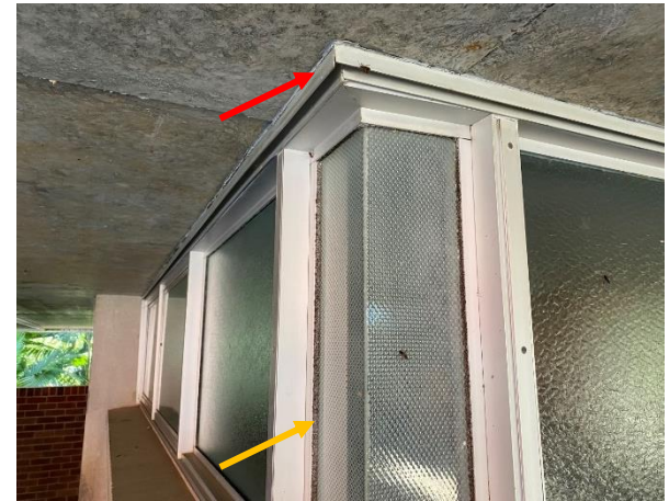
Photo 18: Building E - Asbestos grey putty/filler to top seal of aluminium windows (red) and window mastic with no asbestos detected but consistent with Building B (JBS&G 2021) which reported asbestos present (orange).
