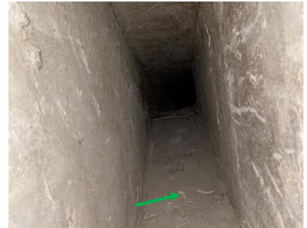
Photo 12: Building A - Non-asbestos render material to internal surface of fireplace flue to Second level of Building A
