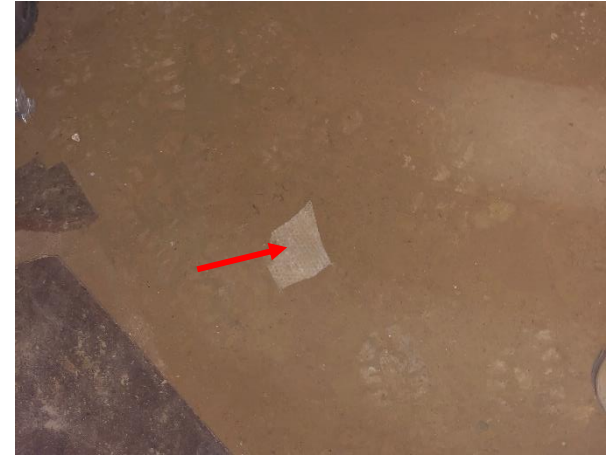
Photo 15: Building A - Loose ACM debris to Building A sub floor
