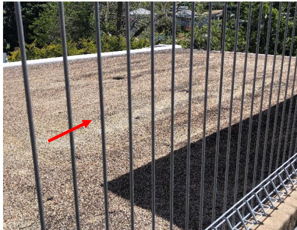
Photo 23: Building E – Suspected asbestos containing waterproofing membrane to pebblecrete roof lining above administration portion. No access available.
