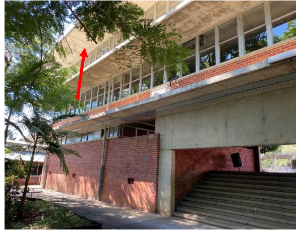
Photo 26: Assumed asbestos containing flat sheet eave linings to northern extent of second level
