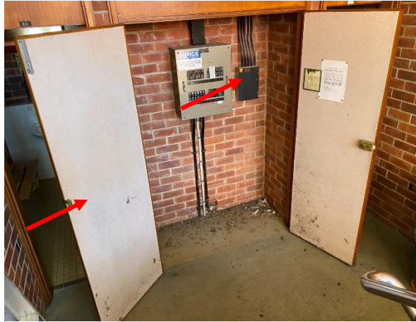
Photo 20: Building E – Asbestos flat sheet internal door linings and asbestos resinous backing board to ER2011
