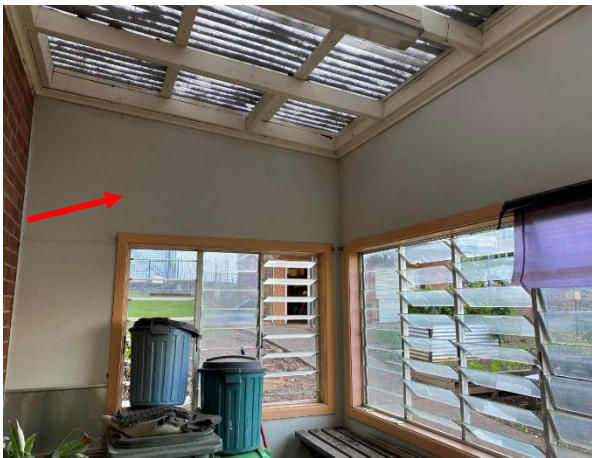
Photo 34: Building AY – Asbestos flat sheet wall linings to AYR0004
