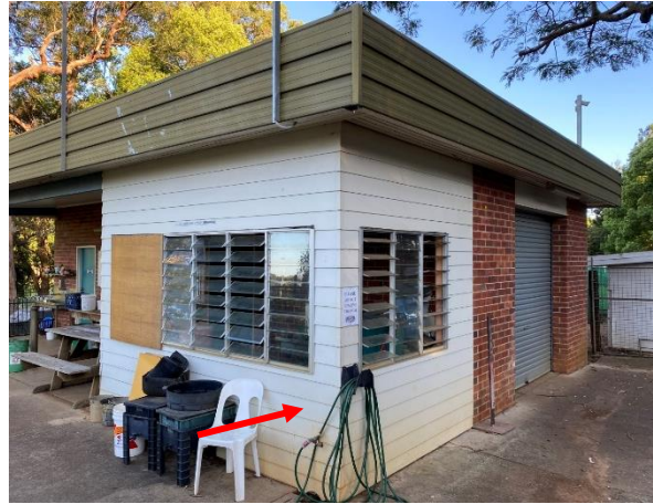
Photo 32: Building AY – Asbestos white weatherboard cladding to NW exterior
