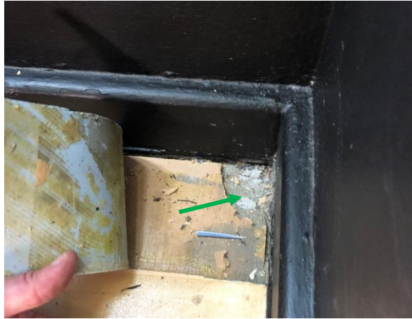
Photo 8: Building A - Non-asbestos fibre board lining beneath vinyl floor sheet and fibre board to AR0019
