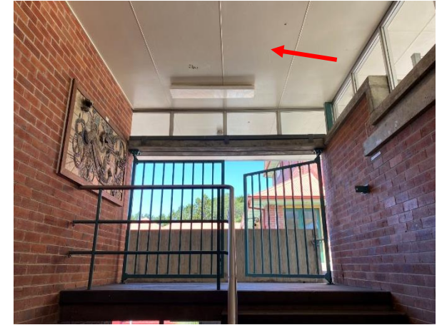
Photo 27: Asbestos containing flat sheet ceiling lining to ER201
