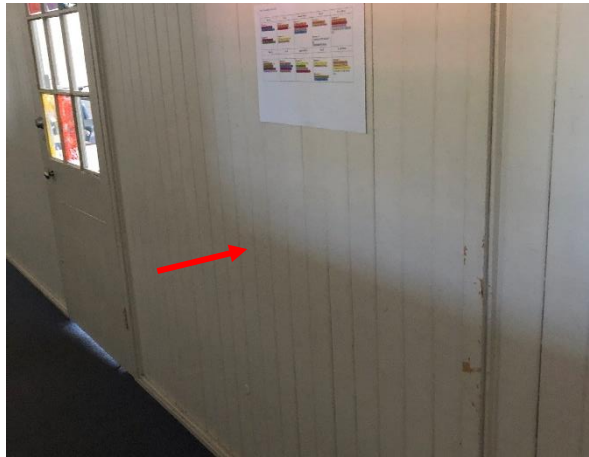
Photo 11: Building A - Lead based white painted walls to AR1014
