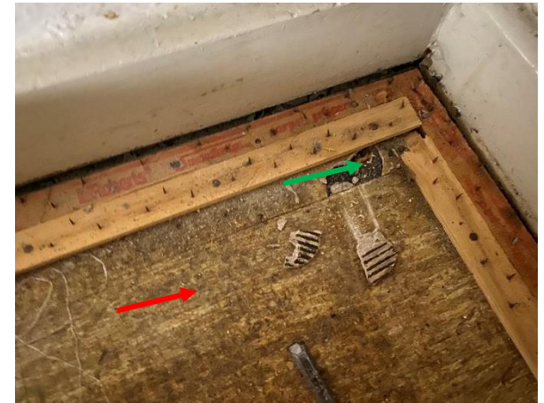
Photo 6: Building A - Asbestos containing vinyl floor tiles with non asbestos (black) adhesive found throughout Building A beneath carpeted floors
