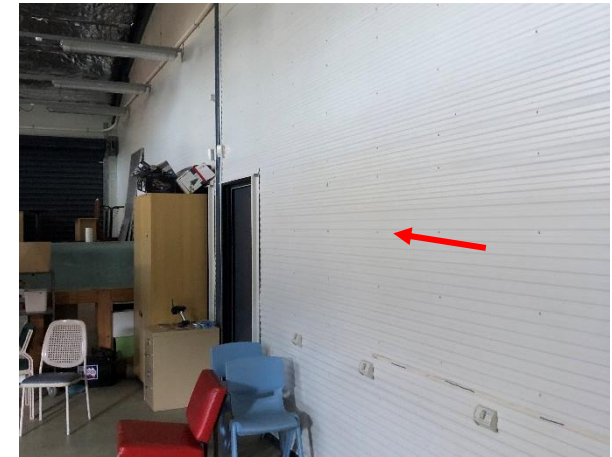
Photo 30: Building F – Suspected SMF internal insulation to dividing wall
