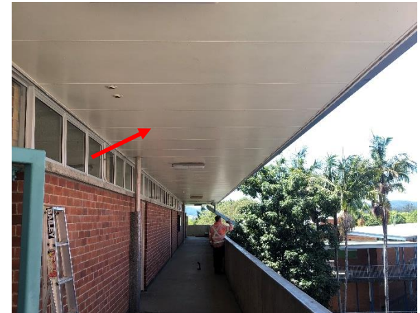
Photo 24: Building E – Asbestos containing flat sheet ceiling lining to ER2015
