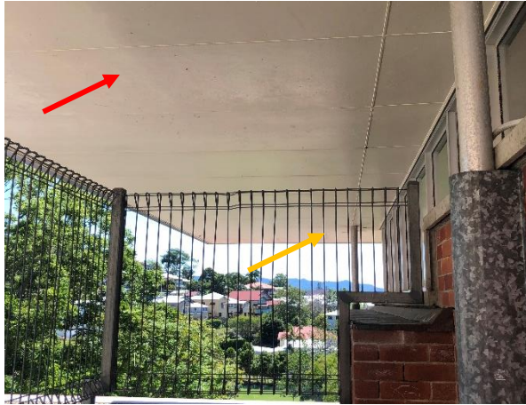
Photo 25: Building E – Asbestos containing flat sheet ceiling lining to ER2017 (red) and assumed asbestos containing flat sheet eave linings to northern extent of second level (orange)
