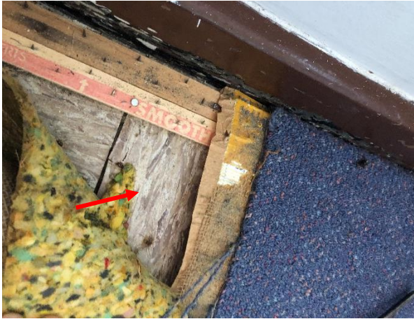
Photo 7: Building A - Asbestos containing vinyl floor tiles with non asbestos (black) adhesive found throughout Building A beneath carpeted floors
