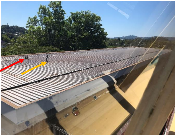
Photo 22: Building E – Asbestos ventilation pipes from basement level (red arrows) and additional suspected asbestos pipe (orange) to roof lining
