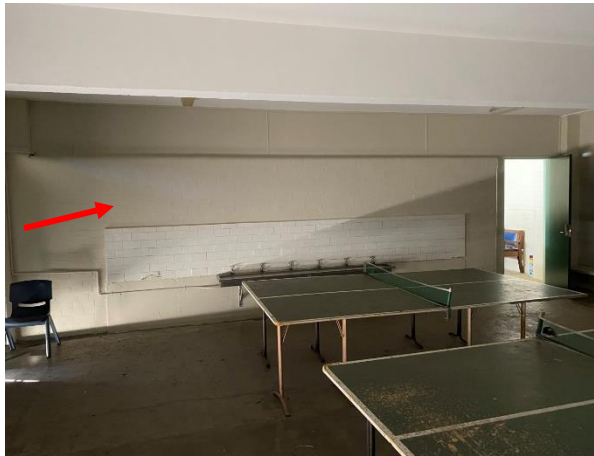
Photo 4: Building A - Example of cream lead based painted walls to Building A Basement level (AR9007 shown)
