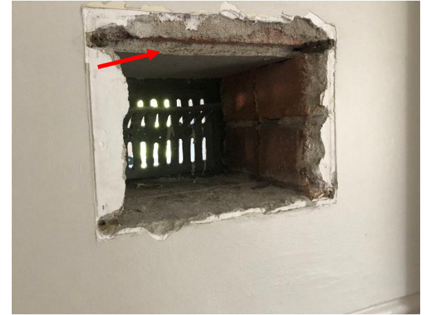
Photo 9: Building A - Asbestos fibre board to top of cross ventilation points along southern hallway (AR1014) to second level of Building A.
