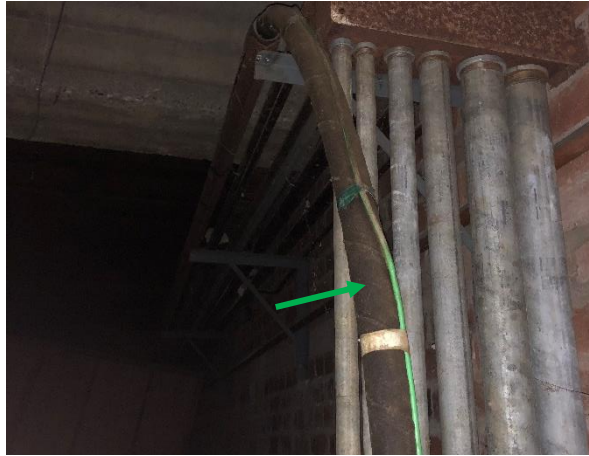
Photo 14: Building A - Non-asbestos bituminous cable sheathing to Building A sub floor
