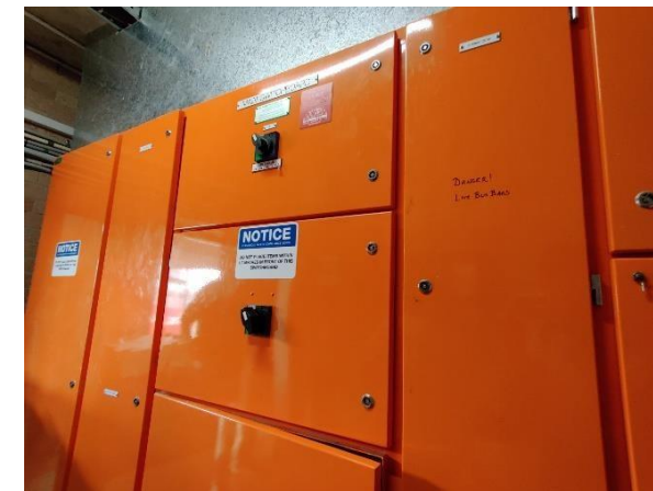
Figure 5: Existing Electrical Main Switchboard
