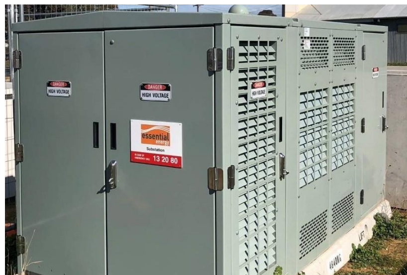
Figure 7 – Typical Essential Energy Substation
