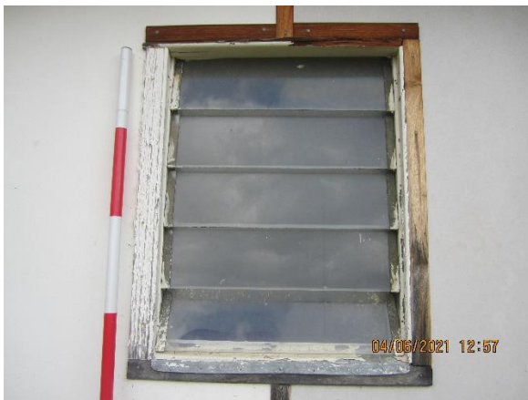
Plate 3-36. Deterioration around the windows and example of the condition of one of the accommodation buildings.
