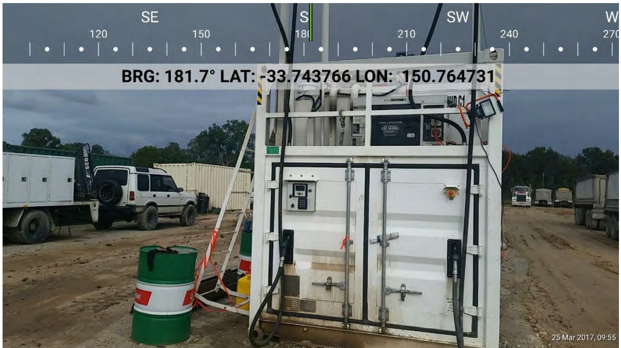
65 Dunheved Circuit, St Marys – RCA Trucks diesel AST and oil drum storage - 2017
