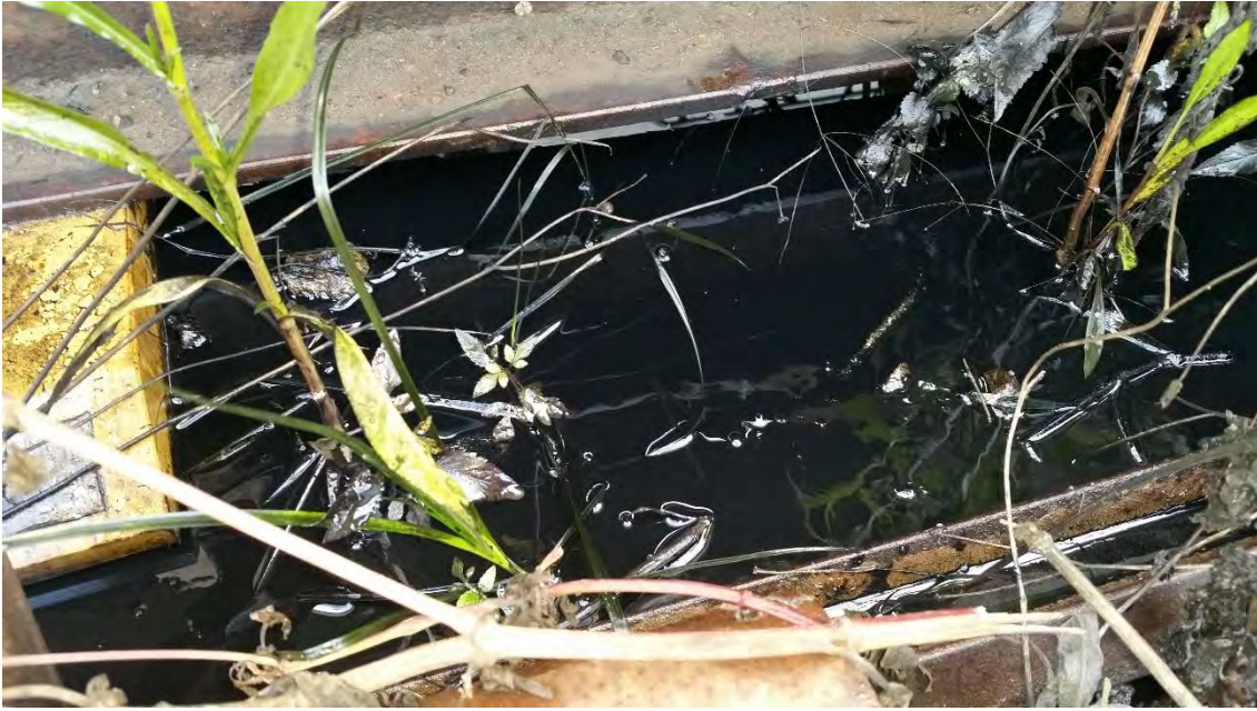
Dunheved Circuit, St Marys – Oily Residue ANTQIP - 2017
