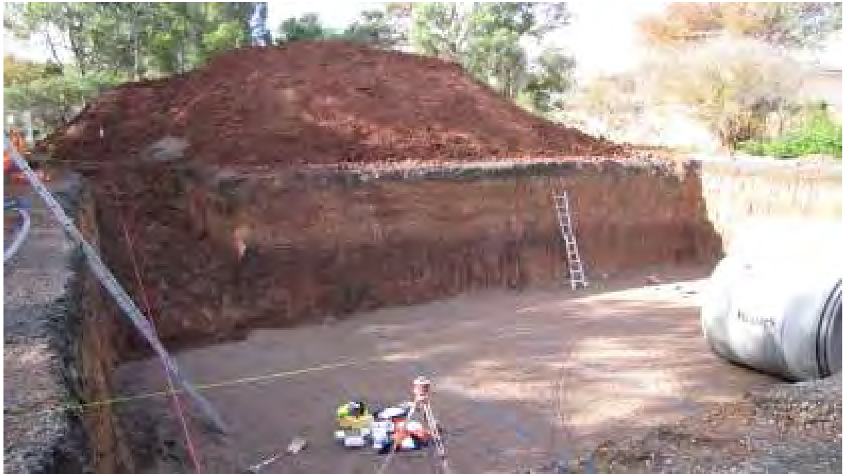
Deep soils of Glenhaven HGL on lower slopes – deep, red clay soils of weathered Ashfield Shale on lower slopes of HGL, as seen in excavated rainwater tank pit (>5m deep) within grounds of Ryde TAFE. (Photo: DECCW/Marion Winkler).
