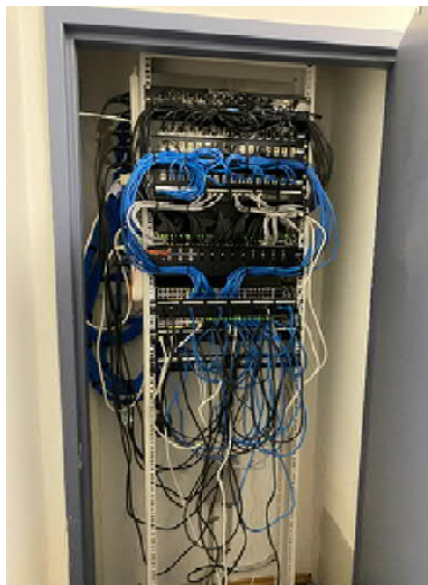
Existing Block B Comms Rack
