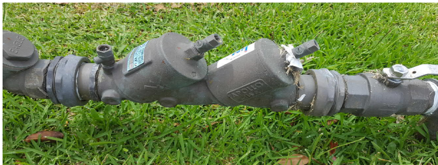
Existing 32mm Backflow Valve Presumed for Irrigation
