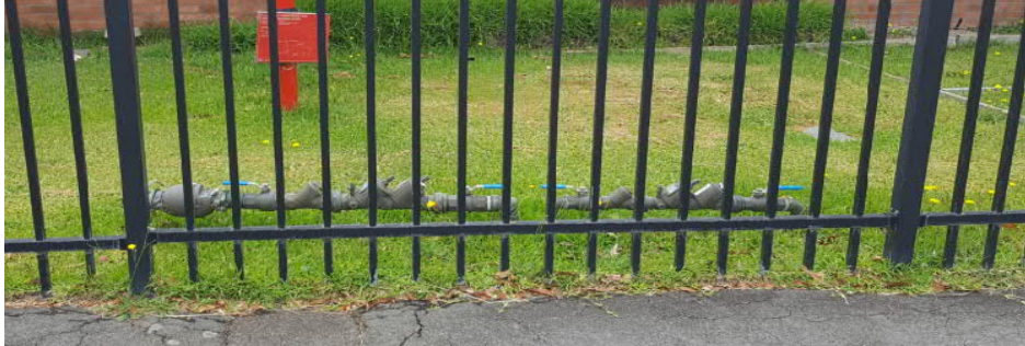
Union Street Water Services Connections
