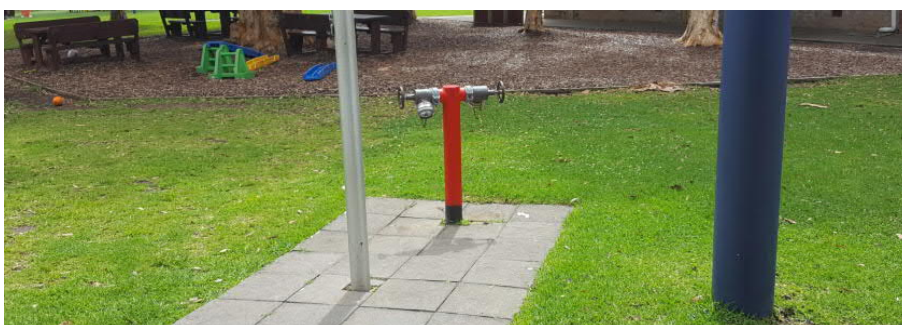
Solitary Double Hydrant Standpipe in Main Courtyard
