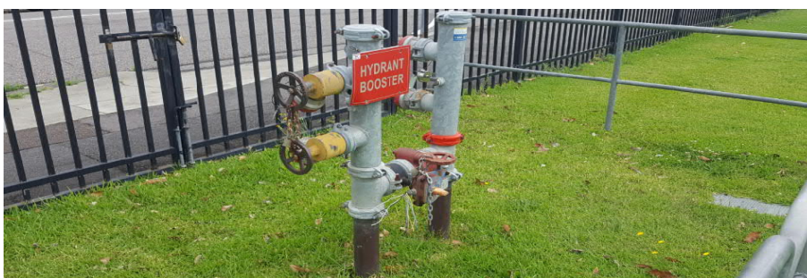
Fire Hydrant Booster Valve and Suction Points
