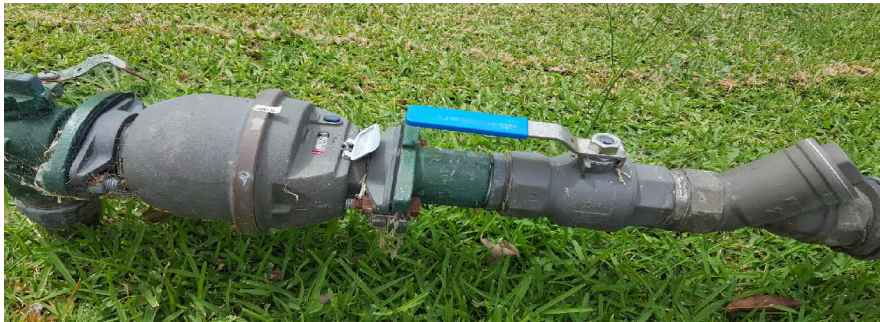
Existing 50mm Water Meter Assembly and Backflow Valve
