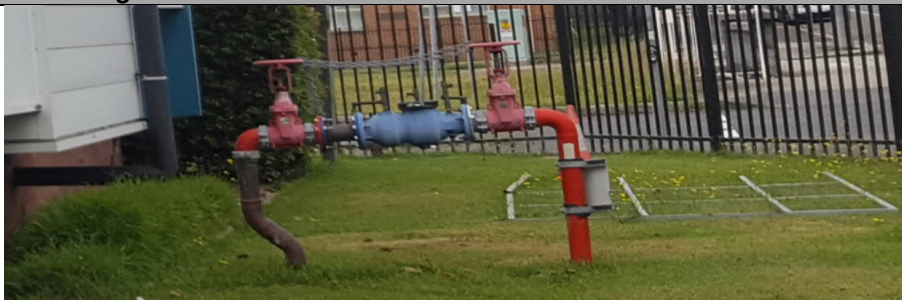
Fire Hydrant Backflow Prevention
