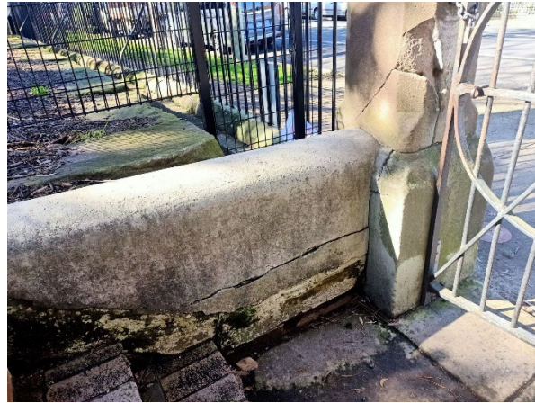
Figure 4.12: Condition of Former Crows Nest House, secondary entrance gates from Bay Road. Source: Curio, 2021.
