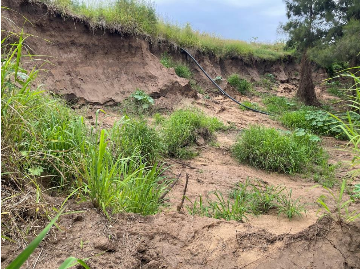
Figure 11: Recent bank erosion due to flooding at HVO12 on the Hunter River (photo taken during January 2022).
