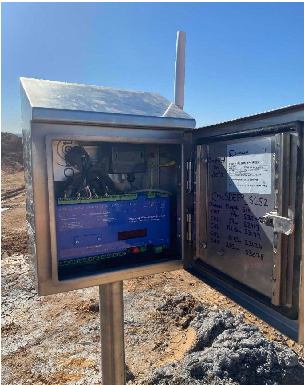
Figure A 2.4 telemetric VWP showing labelled cables (VWP CHESDEEP_S152 shown)
