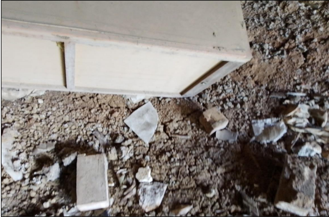
Photograph 11 - Fragments of bonded PACM on ground surface beneath building at 84 Menangle Road.
