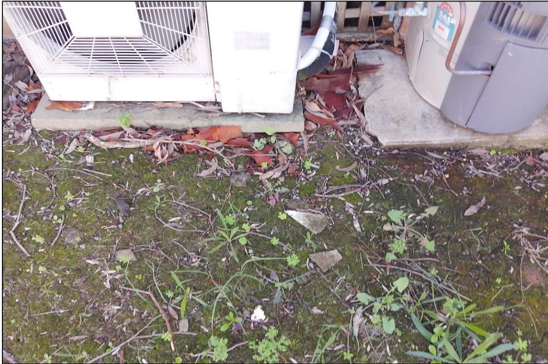
Photograph 9 - Fragments of bonded PACM on ground surface of southern side of building at 82 Menangle Road.
