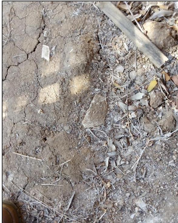
Photograph 8 - Fragments of bonded potential asbestos containing material (PACM) on ground surface beneath building at 82 Menangle Road.
