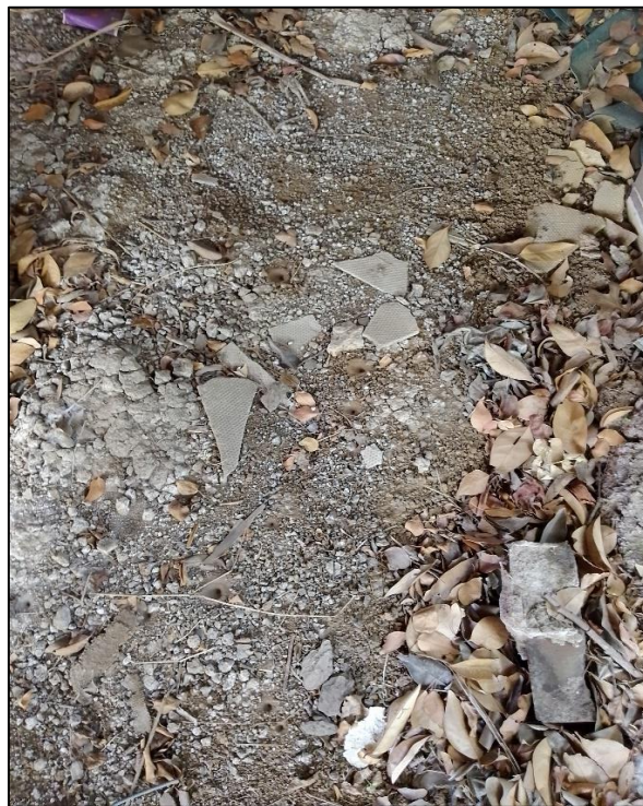
Photograph 14 - Fragments of bonded PACM on ground surface beneath building at 86 Menangle Road.
