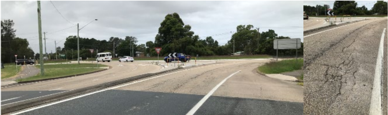
Photograph 7: Rhyolite roundabout at Salt Ash 20-1-2021 in poor condition.
