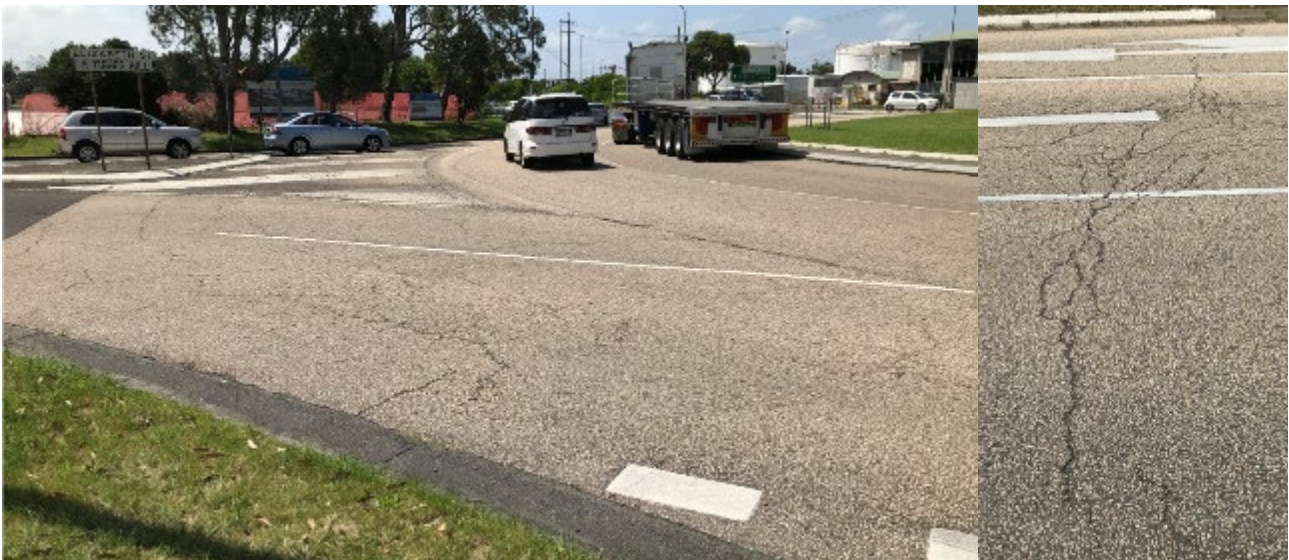
Photograph 8: Rhyolite roundabout at Tighes Hill 3-2-2021 in poor condition.
