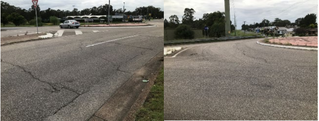
Photograph 10: Rhyolite roundabouts on Victoria Street and Northcote Street, Kurri Kurri in poor or deteriorating conditions on 16-3-2021.
