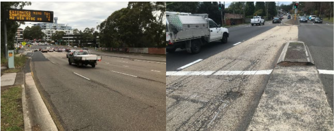
Photograph 16: Rhyolite intersection Pacific Hwy A1, Pymble in poor condition and a Rhyolite turning lane, Warringah Road Forestville in poor condition (24-6-2021).
