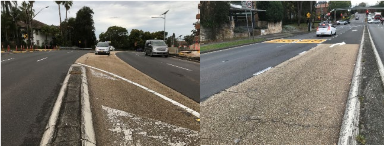
Photograph 15: Rhyolite turning lane Pacific Hwy A1, Wahroonga 24-6-2021 in poor condition.
