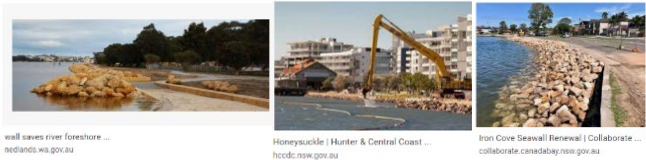
Figure 2: Various rock types used for armour rock (photos from various websites).
