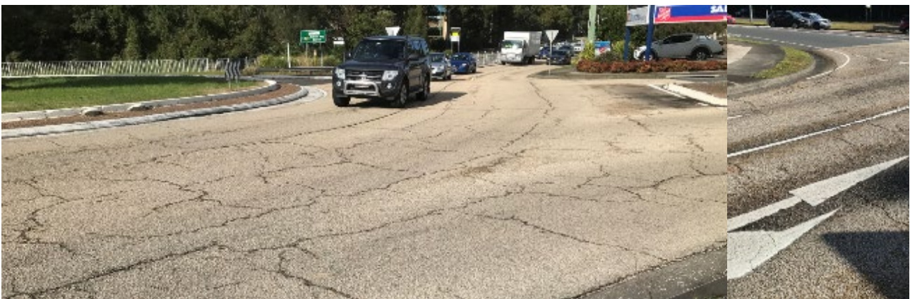
Photograph 9: Rhyolite roundabout at Warners Bay 11-6-2021 in poor condition.
