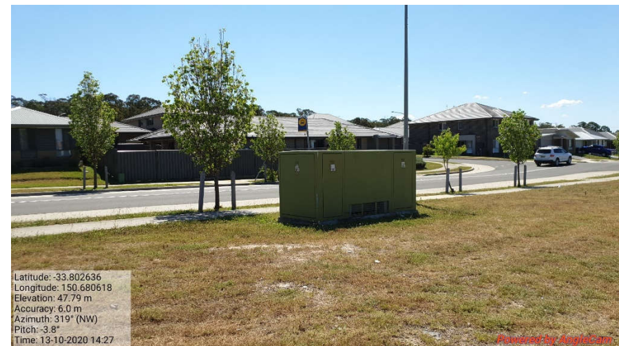
Photograph 4: Substation kiosk along western boundary
