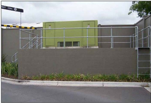
Figure 51 - Example substation raised above 1:100 flood level
