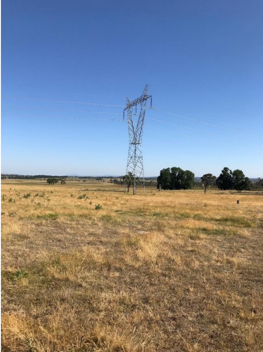
FIGURE 13 TYPICAL STEEL LATTICE TOWER STRUCTURE
