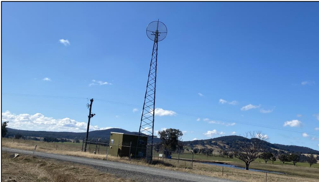
Figure 10 Existing telecommunication facility at the intersection of Hazeldene and Winterbourne roads
