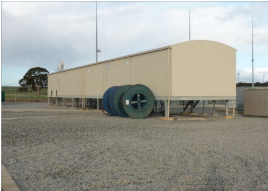
Figure 16 | Typical prefabricated elevated switchroom building
