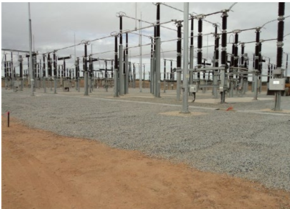
Figure 15 | Typical Outdoor switch gear
