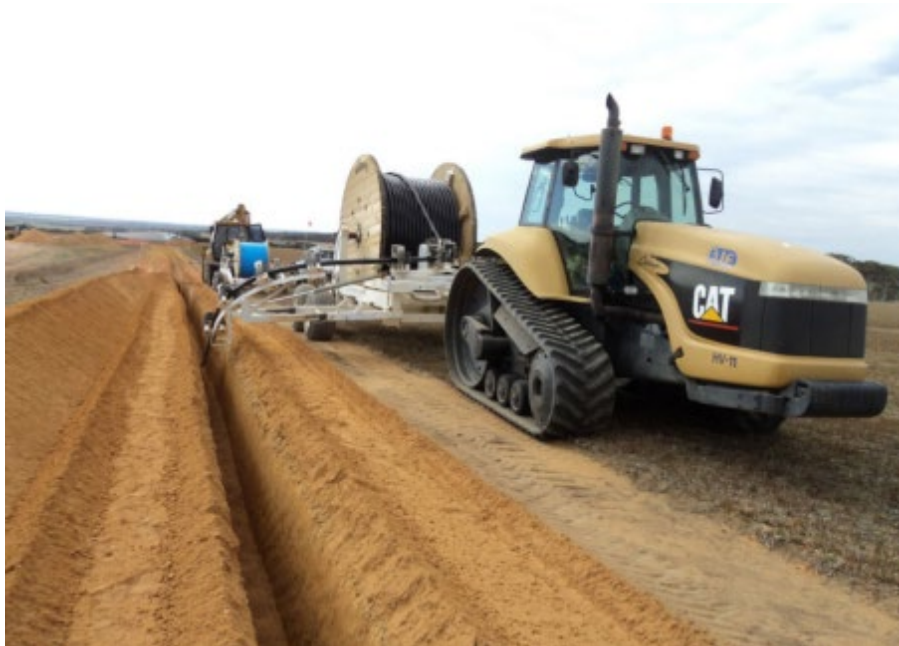
Figure 9 | 33 kV underground cabling
