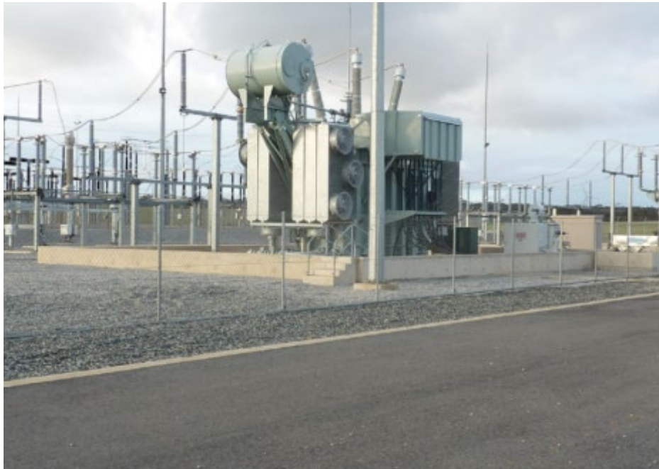
Figure 14 | Typical Wind farm main and neutral earth transformers
