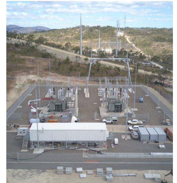
Image 4: Typical Substation (Source: Vestas)
