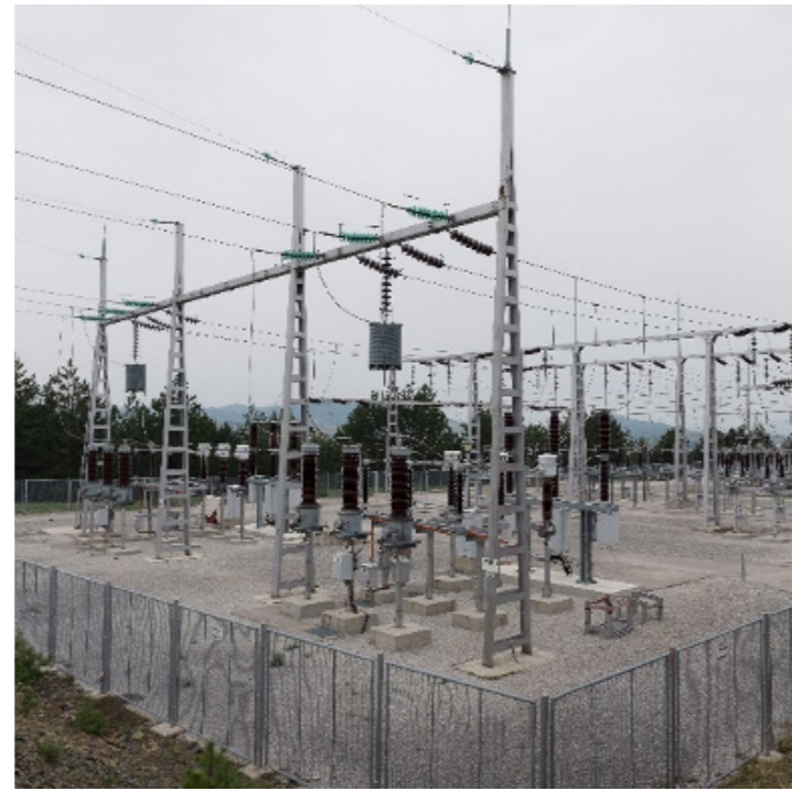
Image 2: Switchyard (Source: ERM)
