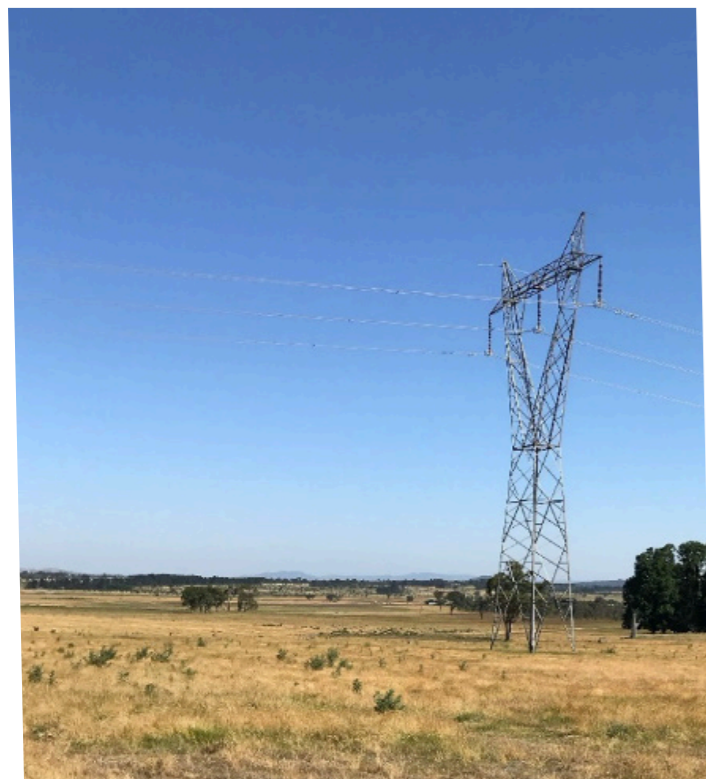
Image 32: Transmission Line (Source: Vestas)
