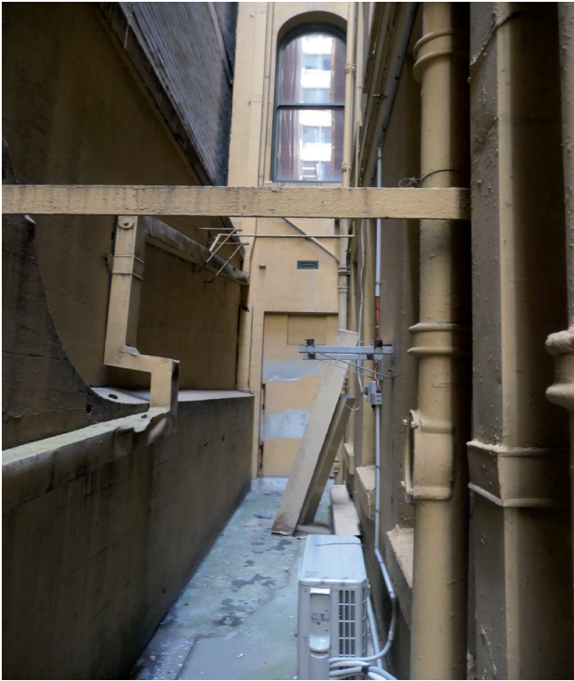
Figure 3.20 An air-conditioning condenser unit in the southern 'Area' Source: GBA Heritage, 2020
