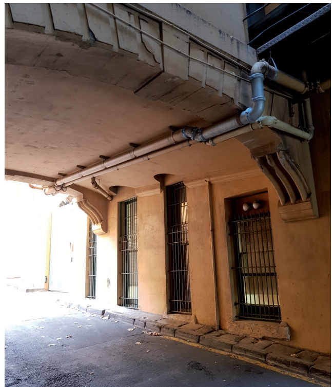
Figure 3.23 Looking to the north side of the heritage building from Phillip Lane, showing the damaged and broken windows sills. Source: GBA Heritage, 2020
