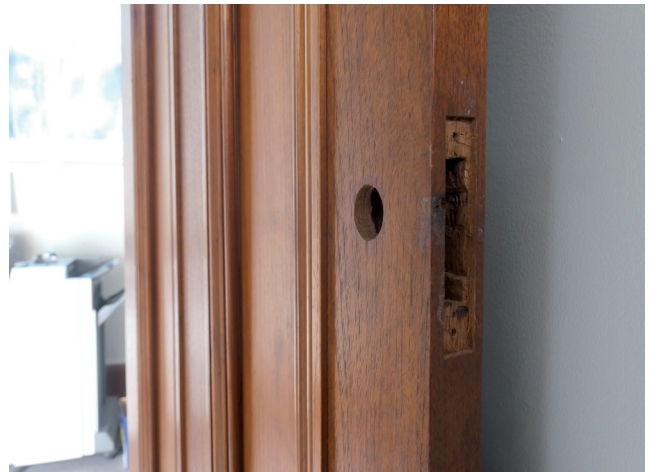
Figure 3.81 A door with missing furniture on level 6 Source: GBA Heritage, 2020
