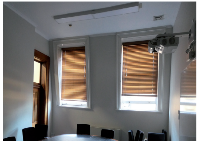
Figure 3.66 Typical mounted projector installed in an office space on level 6. Source: GBA Heritage, 2020
