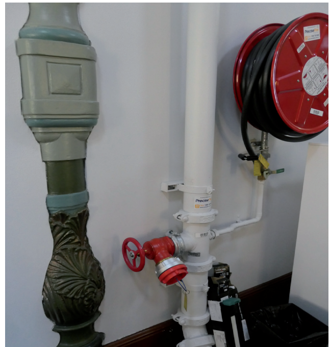
Figure 3.61 Typical fire hose reel and hydrant throughout the building on all levels Source: GBA Heritage, 2020
