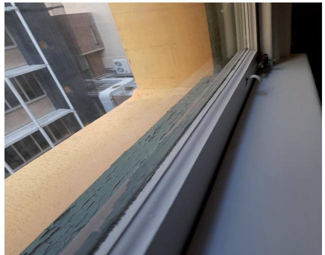
Figure 3.89 Cracking and flaking of the paintwork to the exterior sill level of window on level 4. Source: GBA Heritage, 2020
