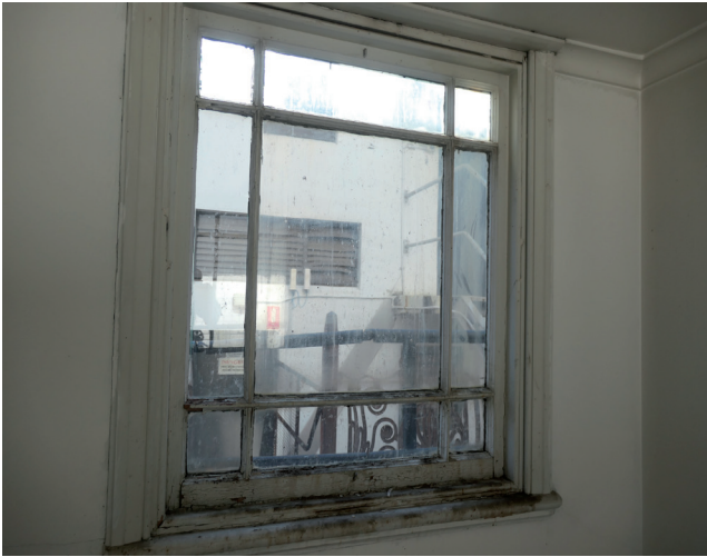
Figure 3.90 Cracking and flaking of the paintwork to the exterior sill level of window on level 6. Source: GBA Heritage, 2020
