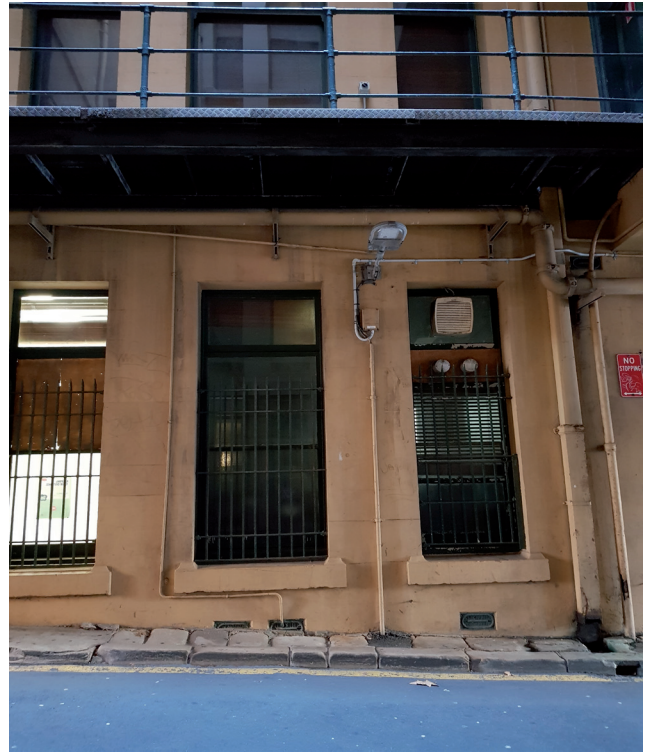
Figure 3.22 Looking to the north side of the heritage building from Phillip Lane, showing the louvre vents are hidden under the finished floor level. Source: GBA Heritage, 2020
