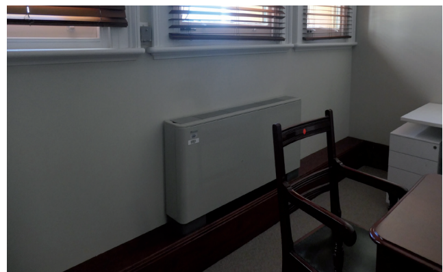
Figure 3.60 Typical floor standing split systems throughout the building Source: GBA Heritage, 2020
