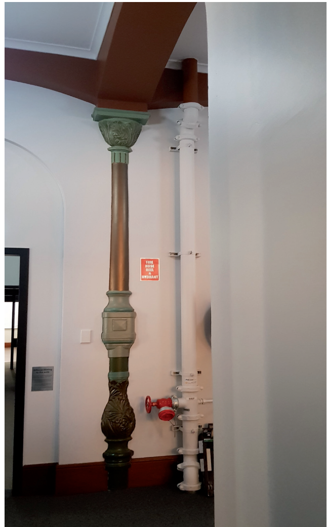
Figure 3.47 Cast iron column to the former open stair embedded into the north wall on levels 2-5. Source: GBA Heritage, 2020
