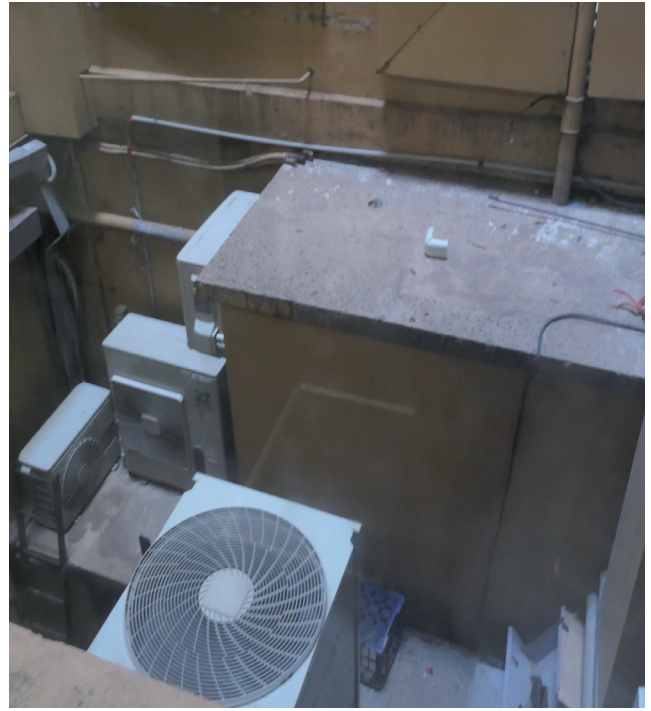
Figure 3.36 Air conditioning condenser units located in the central light well Source: GBA Heritage, 2020
