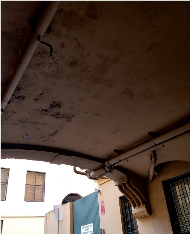
Figure 3.27 Flaking and peeling of paintwork over Phillip lane. Source: GBA Heritage, 2020
