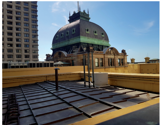
Figure 3.15 General view of the roof to the north, showing the copper roof sheeting that generally look in good condition. Source: GBA Heritage, 2020
