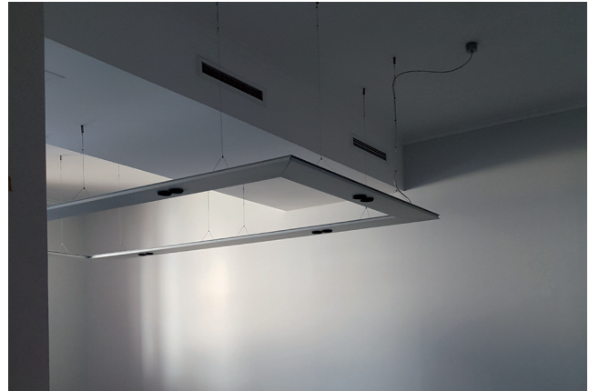
Figure 3.59 Typical exposed air conditioning duct throughout the building Source: GBA Heritage, 2020
