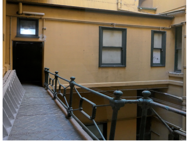
Figure 3.42 The original walkway to lozenge-shaped over Phillip Lane on level 3 Source: GBA Heritage, 2020
