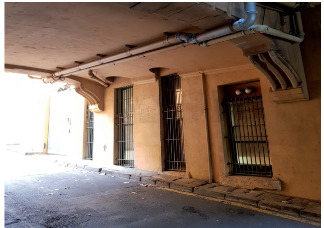
Figure 3.32 North side of the building over Phillip Lane, showing the buried and damaged window sills. Source: GBA Heritage, 2020
