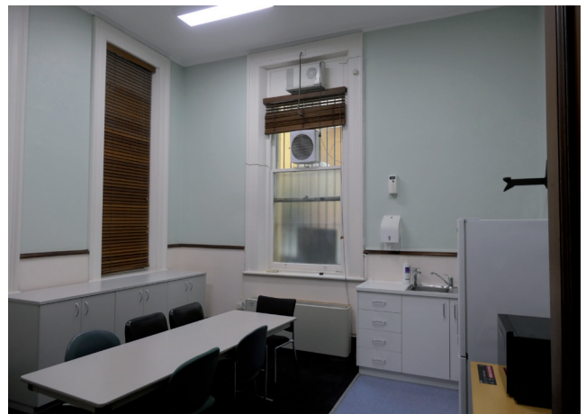
Figure 3.46 A kitchenette on the first level, showing vents and mechanical fans installed within the window sashes Source: GBA Heritage, 2020
