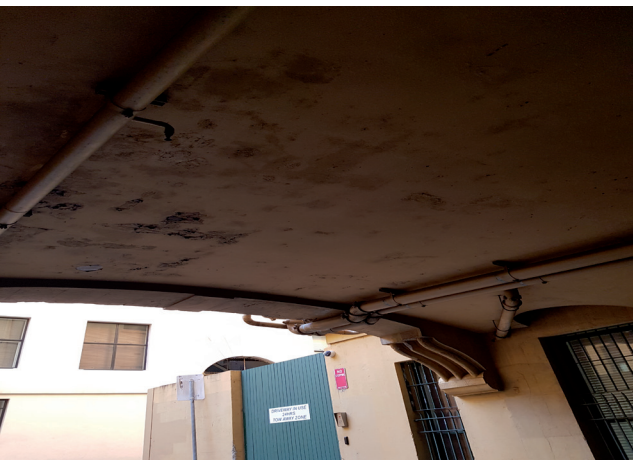
Figure 3.33 Flaking paint of the archway ceiling over Phillip Lane. Source: GBA Heritage, 2020
