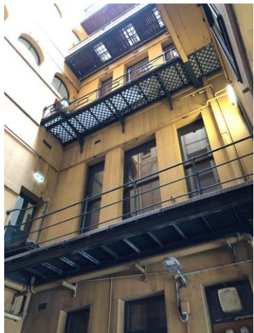
Phillip Lane Lightwell at the northern end of the site looking south
