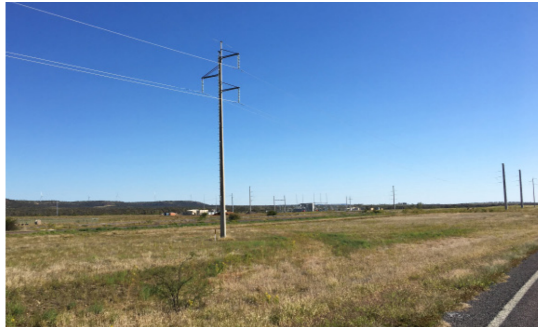
Image 4 Transmission Line (Source: NGH)
