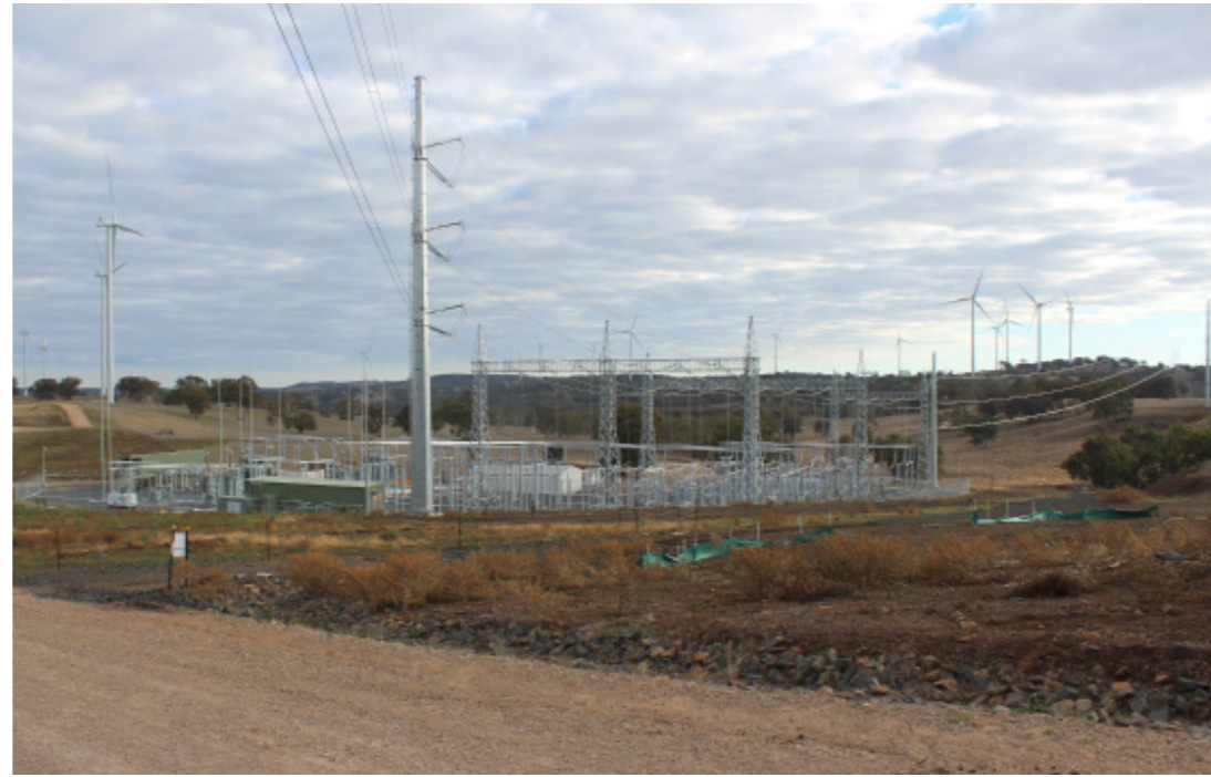
Image 2 Typical Substation (Source: NGH)
