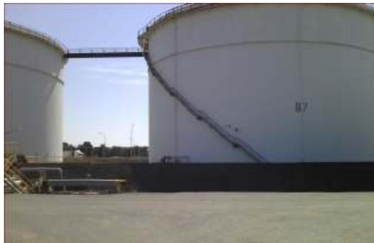
Image 4 - Example of Bund around Fuel Tanks
